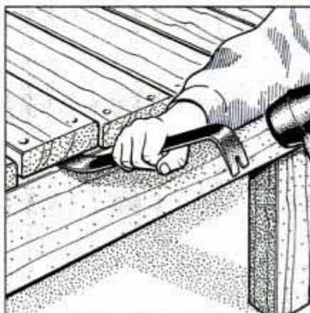
8 Then, use a pry bar to remove both pieces. Cut each at the joist positions and reinstall. Then install a filler piece.
