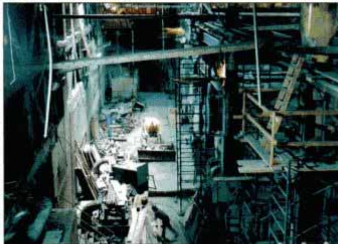
Ground zero, a month later. Debris still litters level B5 while new floors take shape to the right, above damaged refrigeration plant.
