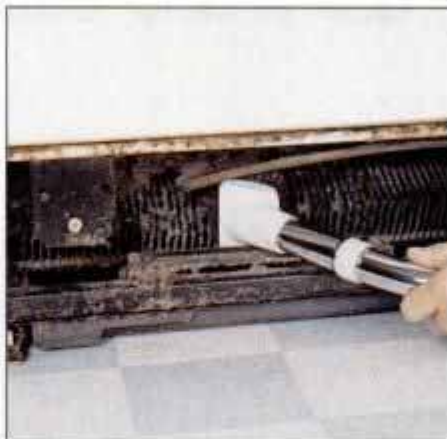
2 Use a vacuum cleaner to pull the matted dust from the coil. If necessary, clean the tubes with degreaser.
