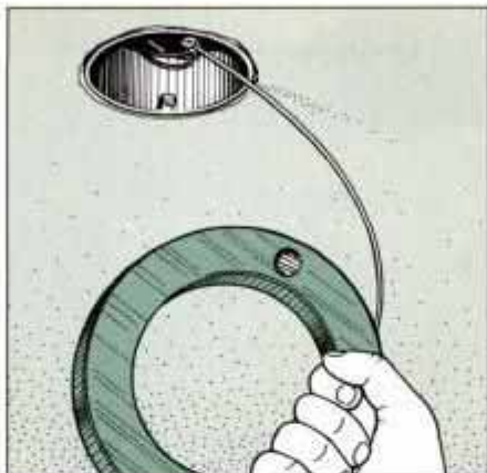
18 Feed the fish tape through the ceiling fixture and push it through the ceiling cavity to the cable.
