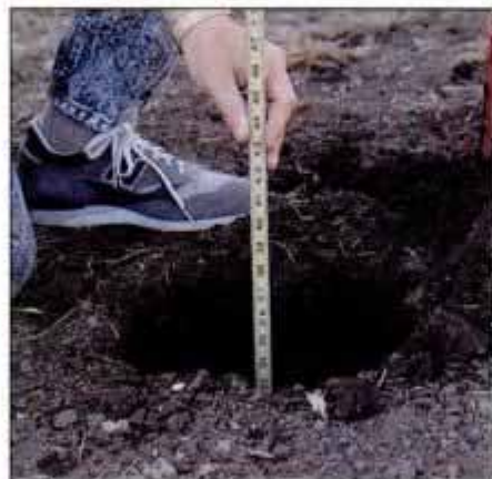
2 Use a tape measure to check that the hole extends below the frost line. Codes vary, but a 36-in.-deep hole is common.
