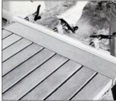
15 Place a long scrap block against the top frame rail while gluing and clamping the slats to the rails.
