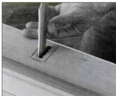
7 Finish the apron mortises with a sharp chisel. Pare down to flatten the mortise sides and square the mortise ends.
