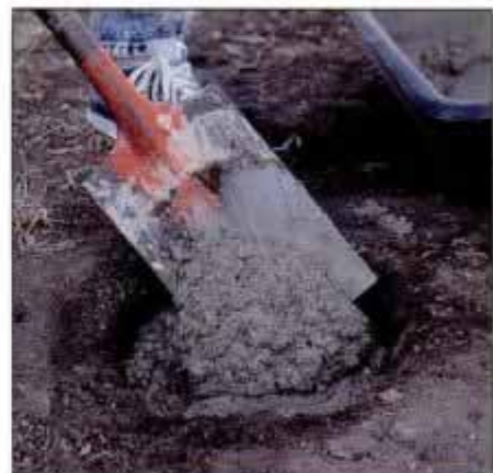
3 Mix premixed concrete in a wheelbarrow and shovel it into the hole. Two bags should handle one 36-in. hole.
