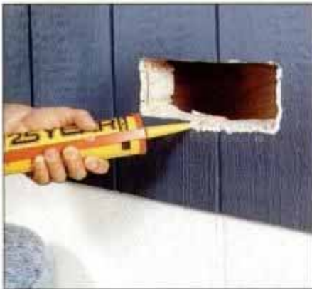
4 Once the opening is cut, check the faucet for fit. When satisfied, apply a bead of caulk to the rim of the opening.
