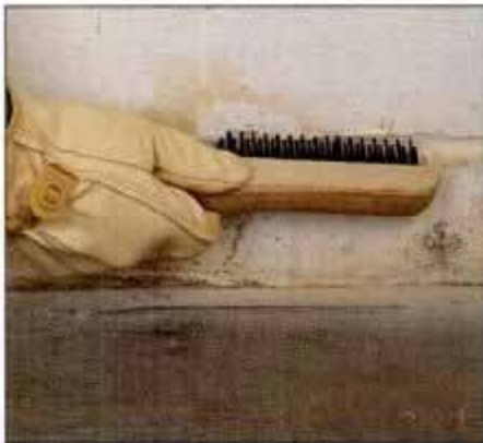
3 Remove any blistered paint from the interior of your foundation wall with a wire brush and coarse sandpaper.
