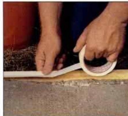
3 Install a form board against the side of the slab. Then cover the board with masking tape to keep patch from sticking.
