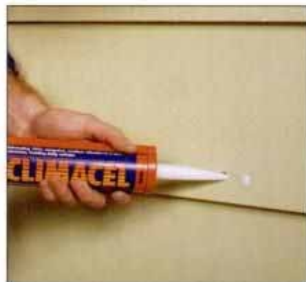
5 Fill any holes, like these that were left when a phone line was moved. Keep caulk flush with the surrounding surface.
