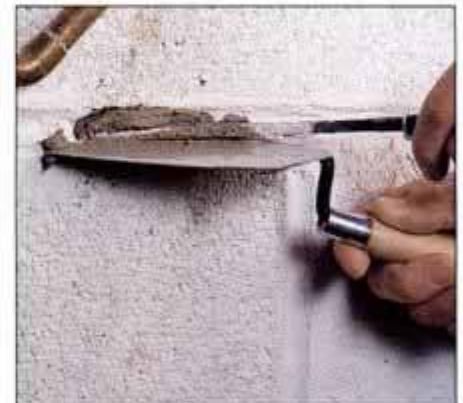
8 Pack fortified mortar into the wall joints using small mason's trowels. Make sure the entire space is filled.
