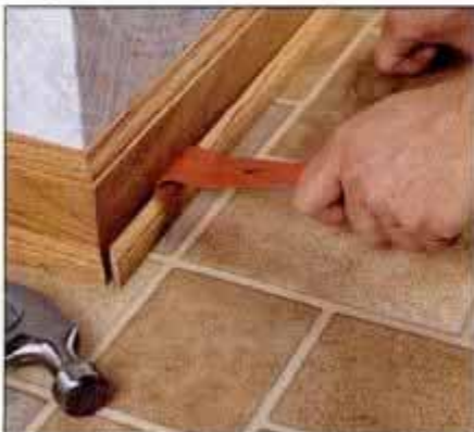
1 Begin floor preparation by removing the baseboard shoe molding with a flat pry bar. Pull nails from the back of board.
