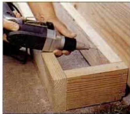
14 Make sure the top of the box is parallel to the top of the deck. Then attach it to the deck with screws.
