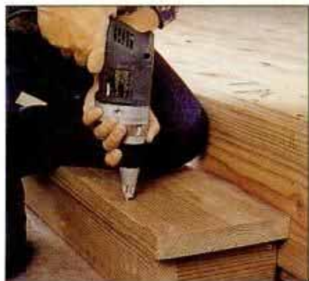
15 Complete the step by installing a tread. Use at least three screws on the sides and several along the front and back.
