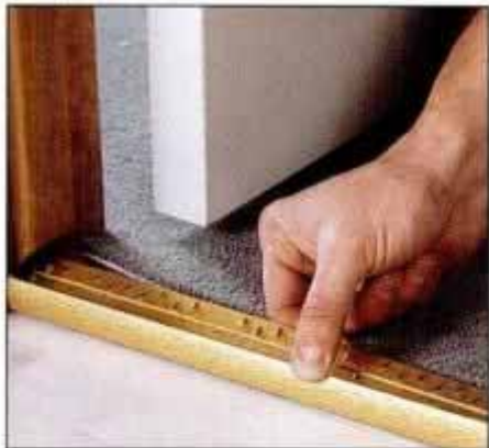
14 When laying vinyl next to carpet, use a metal tack strip. Nail the strip onto the vinyl and bend it over the carpet.
