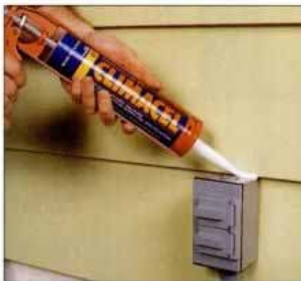
4 Apply silicone caulk around all outdoor electrical fixtures to prevent any water from entering these boxes.
