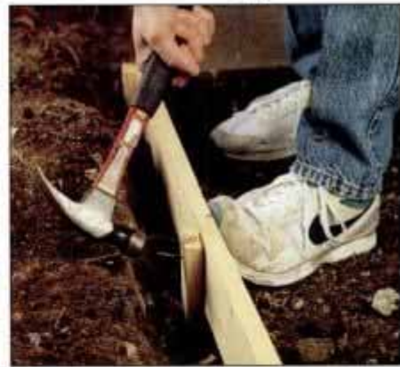
6 To install a new sidewalk section, first break up and remove the old concrete, then build rough 1 × 4 forms.
