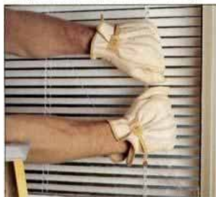
3 When the putty and points are gone, gently remove the broken glass. Be sure to wear heavy gloves to prevent cuts.
