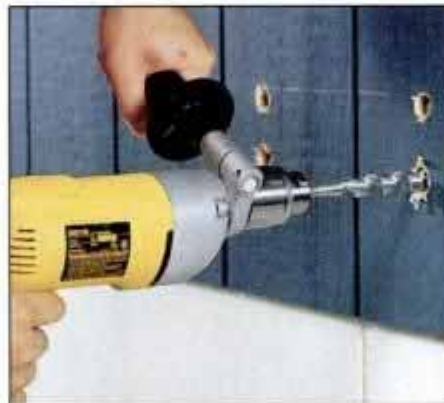
2 Once the cutout is marked, bore saw-blade entry holes at the four corners. Use a \frac{3}{4} -in. bit for good clearance.
