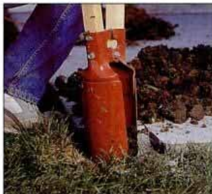
2 Use a post-hole digger to dig pier footing holes below the frost line. Square off the bottoms of the holes.
