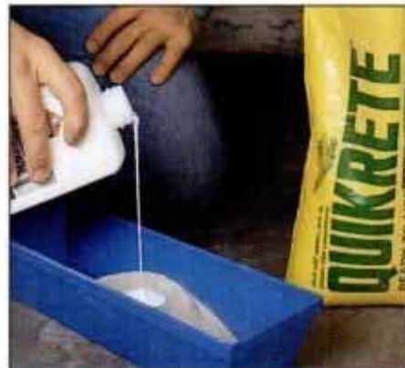
7 Fill any gaps in the foundation's mortar joints with a mixture of premixed mortar, water and a latex bonding agent.
