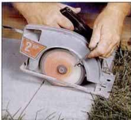
1 Begin by laying out the deck location. If concrete must be cut, use masonry blade in an old circular saw to score surface.
