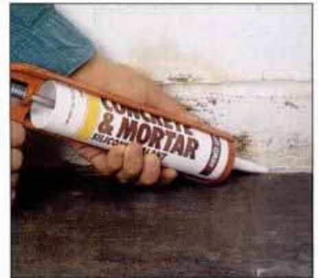
5 Caulk small, leaky cracks with a silicone-mortar caulk. Smooth with a putty knife dipped in mineral spirits.
