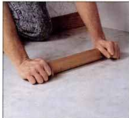
12 Lower vinyl sheet onto adhesive, then roll surface smooth using a flooring roller or kitchen rolling pin.
