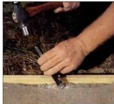
2 On edge cracks or breaks, undercut the edge of the concrete with a cold chisel to increase the bonding surface.
