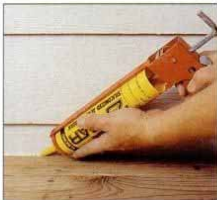
16 To protect the siding behind the ledger from water exposure, seal the top joint with a bead of silicone caulk.
