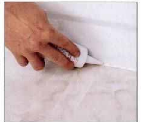
13 Seal around the entire perimeter of the room—and around any plumbing fixtures—with latex tub-and-tile caulk.
