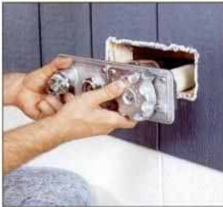
5 Carefully press the faucet into the opening until it seats completely in the caulk. Then brace it in place.
