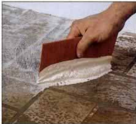
11 Apply vinyl adhesive to the floor with the kit's notched applicator. Cover only half the room at a time.
