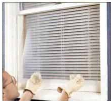
6 Slide the new pane in place from below. Guide it into its upper slot and gently press the bottom against the sash.
