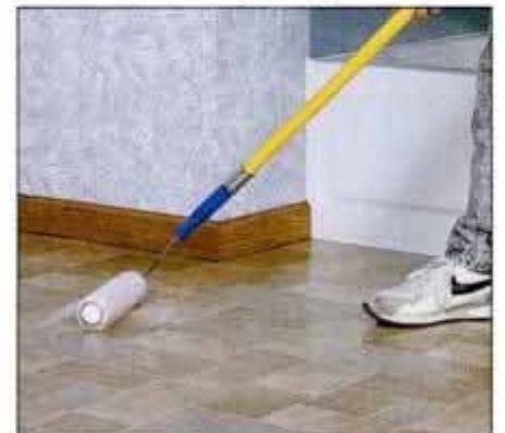
3 For best results, apply an etching solution—using a disposable roller—to deglaze the surface of the old floor.
