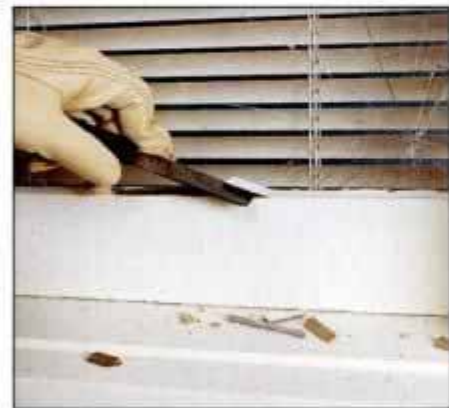
1 Remove the storm window, if necessary, then use a putty knife to pry the old putty from around the broken glass.
