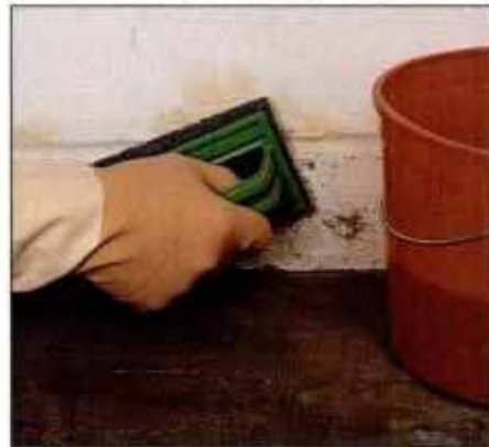
4 Scrub mildew with an abrasive pad and a mix of household bleach and water. Use muriatic acid on efflorescence.
