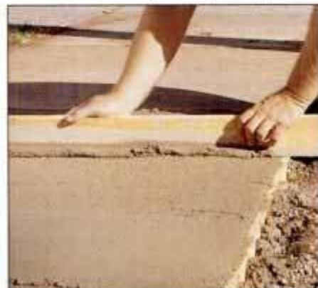
7 Pour the concrete between forms and level the surface by moving a screed board back and forth across the forms.
