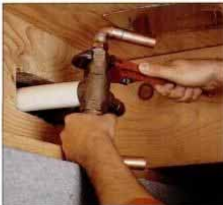
7 Once the soldered turns are joined to the check valves, thread these assemblies into the faucet's valve body.
