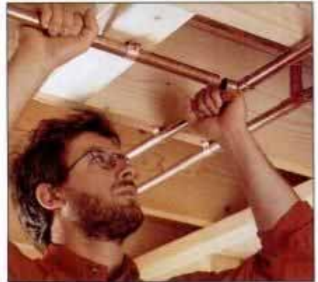
9 Cut into the hot and cold supply lines, and solder tees in place. Then connect the faucet tubing to the tees.
