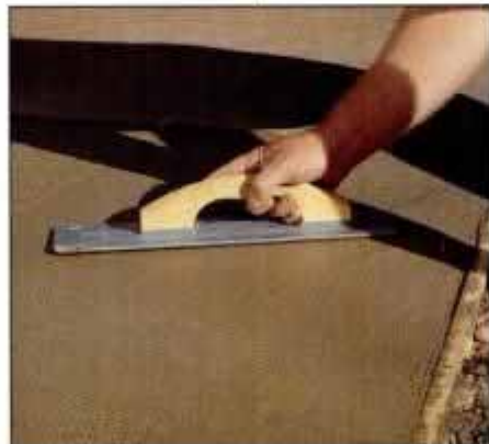
8 When the concrete stiffens, work the surface with a float. Smooth the top until puddles just start to form, then stop.
