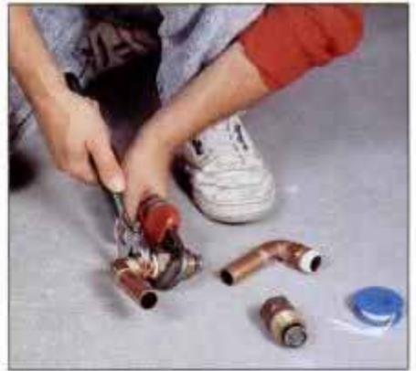
6 Solder copper street ells to stubs and male adapters. Let assemblies cool, then thread them into the check valves.
