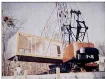
DAY 30. First-floor rear section is hoisted into position. Steel cross banding and 2 x 4s stiffen boxes during transportation.
