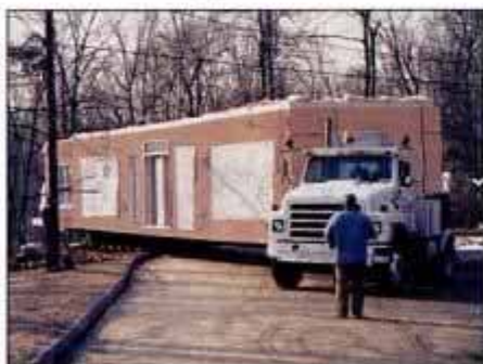
DAY 30. Modular boxes begin arriving by truck. Average box weighs 32,000 pounds. This unit is the first-floor front entry.
