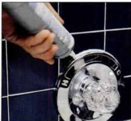
13 Sparingly apply a bead of silicone caulk around the faucet trim plate to keep water from traveling behind the wall.
