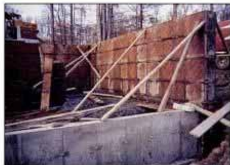
DAY 13. Forms are erected for concrete foundation. Crushed stone provides drainage under slab to help keep basement dry.
