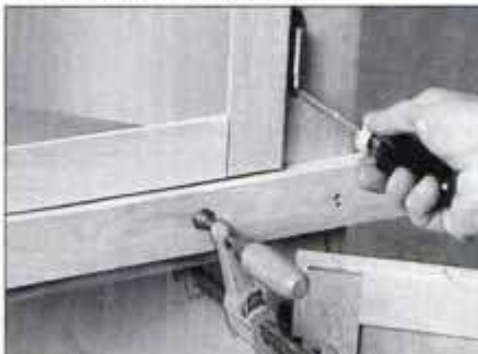
23 Clamp a straight board to the front of the cabinet to support the doors as you screw their hinges to the face frame.
