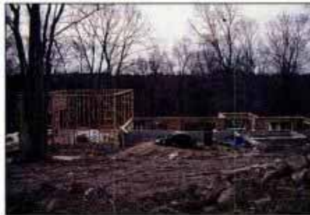
DAY 25. Garage framing is completed. Entire rear portion of house features stick-built construction for full walk-out basement.
