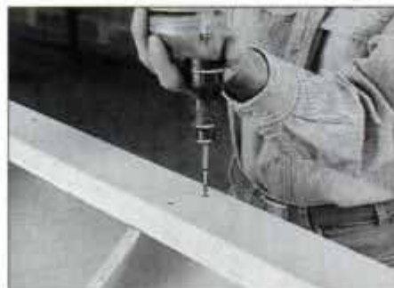
11 Drive screws—through prebored and counterbored holes—from the case back into the back of each shelf.
