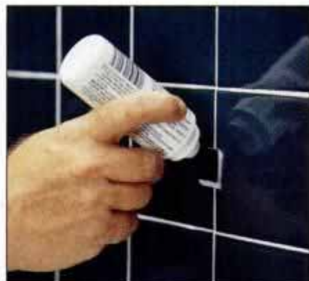
15 After the silicone caulk has cured, seal each grout joint with clear silicone sealer and follow by buffing with a soft, dry cloth.
