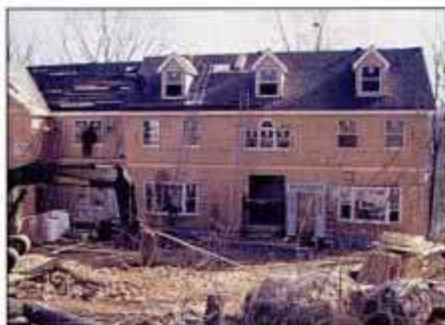
DAY 32. Roof shingles are installed. Dormers come preassembled and are hoisted by crane and installed in precut openings.
