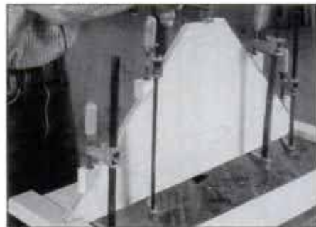
10 Use joining plates and glue to attach the shelves to the face frame. Remove clamping ears later with a chisel.
