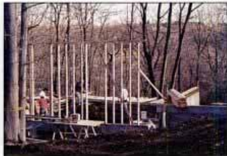
DAY 18. Foundation is stripped and garage is framed for accurate elevation. At this point, house is being built at the factory.
