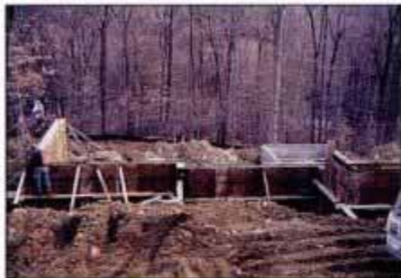
DAY 14. Concrete pouring is completed. Accuracy to elevation and square is maintained to within \frac{1}{16} in.
