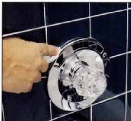
14 Use a facial tissue to wipe all but a narrow bead of caulk from the trim-plate seam, so that caulk will be nearly invisible.
