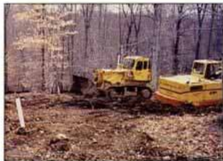
DAY 5. Lot is cleared and excavation begins. Rock ledge is reached 5 ft. down. Fill is brought in to soften slope angle.
