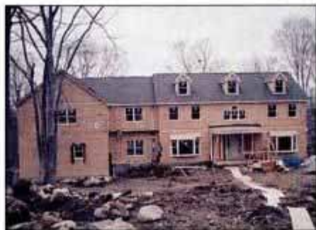
DAY 41. Exterior is just about complete except for siding. Front entry features porch and two bumped-out coat closets.
