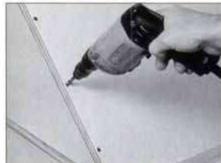
16 Bore pilot holes through the case sides, and attach the case sides by screwing them into the shelf edges.
