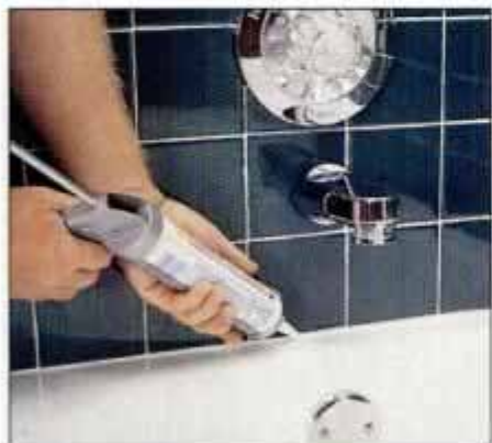
10 Apply silicone caulk to the seam between tub and tile using even pressure and only enough caulk to fill the gap.
