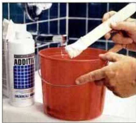
6 Mix powdered grout and a drying-retarder additive to the consistency of toothpaste. Use a clean container.
