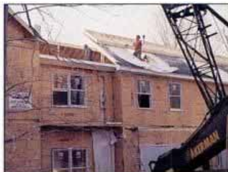
DAY 31. All seven boxes are in place. Roof consists of three hinged sections. Lower section, complete with soffit, flips down.
