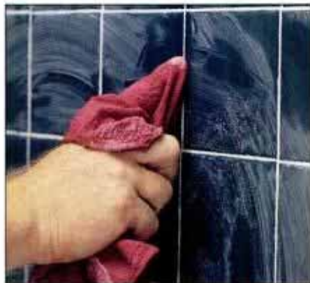
8 Wipe away the excess grout with a damp rag. Then use the rag and your finger to smooth each joint individually.
