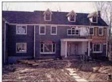
DAY 52. Prestained cedar siding and trim boards are applied. Balance of job includes heating system, flooring and interior work.
