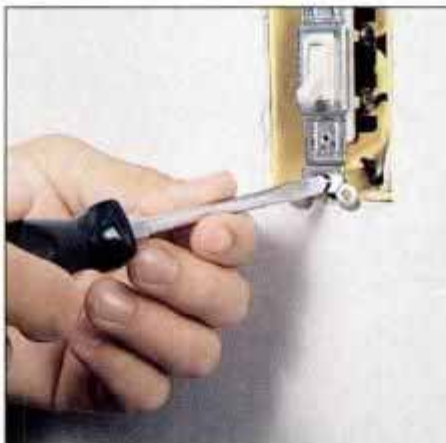
10 Remove the switch's yoke screws and pull the switch out from its box to gain access to the fixture wires.
