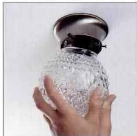
5 To service a flickering light fixture, start by removing the fixture's globe or diffuser. Then, carefully pull the fixture down from the ceiling.
