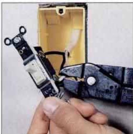
11 Use a multitool or side cutters to cut the wires. To replace 3-way switches, transfer one wire at a time to the new switch.
