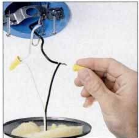
8 Twist stranded fixture wire around the solid circuit wire and thread the twist connector back over them.
