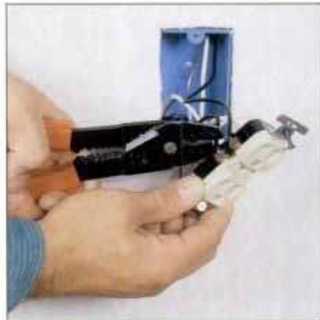
15 Cut the incoming and outgoing black, white and bare ground wires from the defective receptacle.
