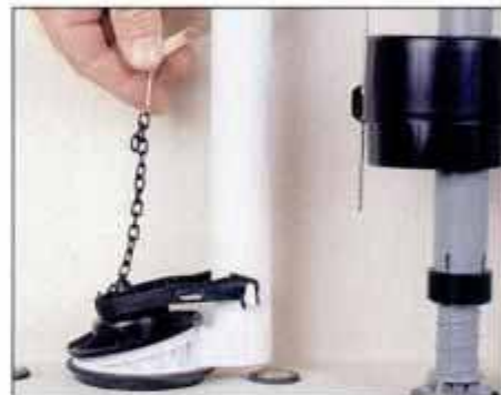
16 Finish installing new flapper valve by attaching the valve chain to the flush lever, leaving about 1/2 in. of slack.
