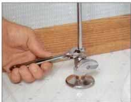
6 Shut off the water at the stop and loosen the supply tube's compression nut before lifting the toilet from the floor.
