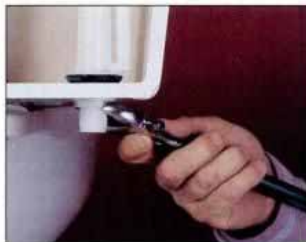
20 Follow by undoing the fill valve's jamb nut with an adjustable wrench to free the fill valve from the bottom of the tank.
