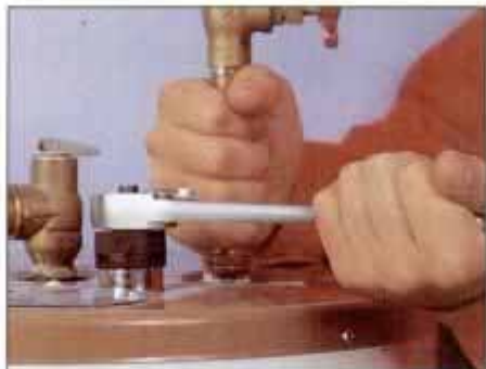
4 To remove a spent magnesium anode rod, first use a 1 1/16-in. socket wrench to loosen the anode rod nut.
