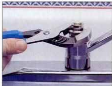
31 Once the handle is off, use a pair of adjustable pliers to loosen the nut that conceals the valve cartridge.
