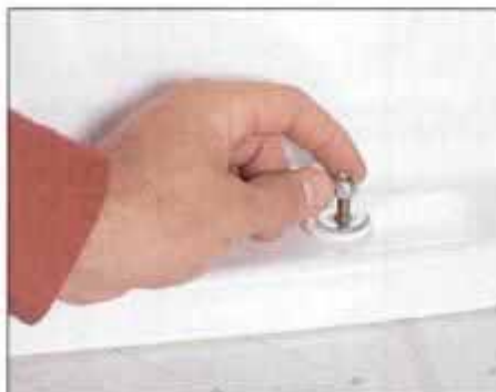
12 Place plastic cap washers, metal washers and chrome nuts on the bolts. Then tighten and saw off excess bolt thread.
