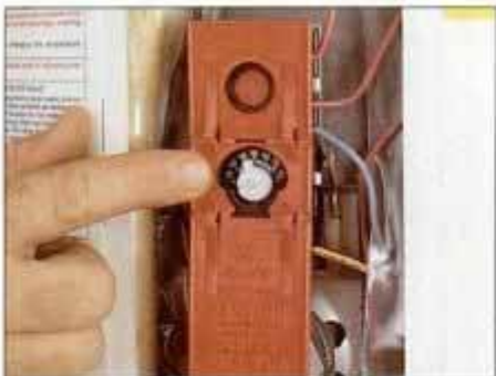
3 The thermostats on an electric heater have temperature indicators and adjustment knobs with screwdriver slots.
