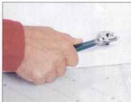
8 Use an adjustable wrench to loosen the closet bolt nuts. Then, lay down newspaper to rest the toilet on after it's removed.
