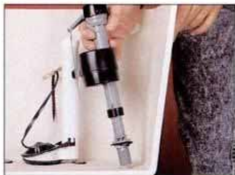
22 Coat new fill valve's washer with pipe-joint compound to form a good seal with tank and insert through tank opening.
