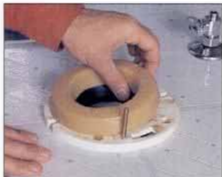
11 New closet bolts make reinstalling the toilet easier. Slide the bolts into the flange slots and press a new wax over the flange.
