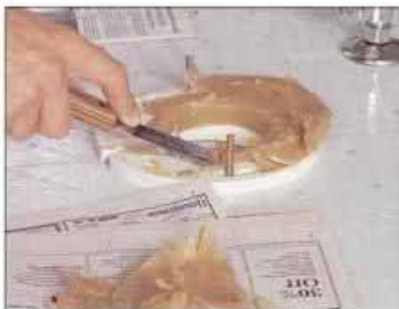
10 Use a putty knife to thoroughly scrape the old wax from the flange. Also check and remove wax from the toilet base.
