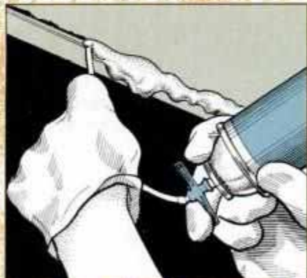
4 Foam caulk is best for sealing large gaps, such as between a window and wall framing. Wear goggles and gloves for safety.
