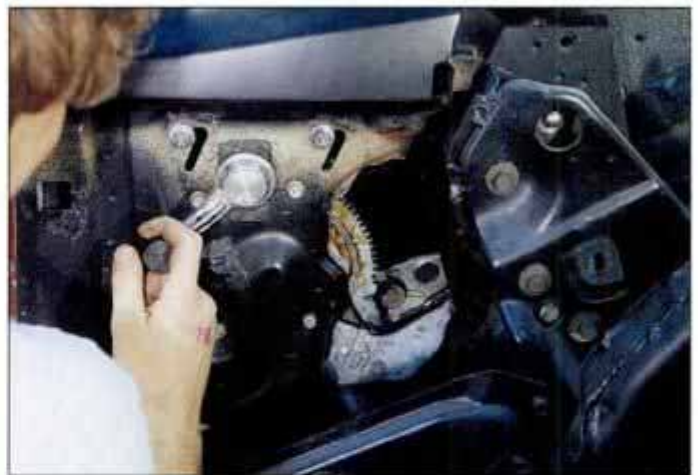
All window mechanisms are repeatedly tested before glass is installed, then tested again before interior trim panels go on.
