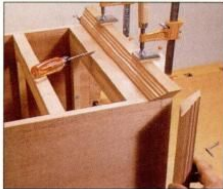
14 Cut base molding to size. Bore pilot holes for screws that join molding and case. Clamp together and drive screws.
