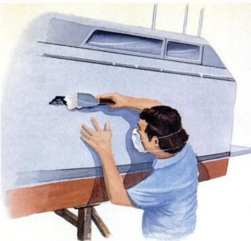
Gouges, cracks or blisters must be carefully patched with epoxy-based fiberglass filler.
