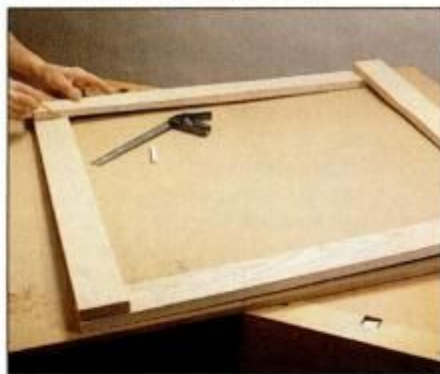
3 Align the top frame members as shown, then mark cutting lines for corner half lap joints directly on the boards.
