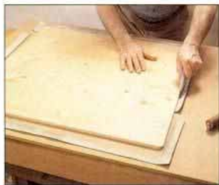
15 Use a roller to smooth the vinyl in place. Then turn over the panel and trim off the excess with a sharp utility knife.
