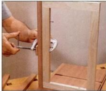
11 Cut frame facing to length and clamp in place. Then tap frame nails into back of facing to create alignment dimples.
