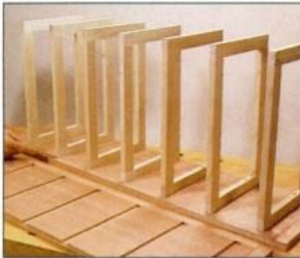
10 Slide all drawer frames into their dados. Then mark on frame edge exactly where frame facing boards should stop.
