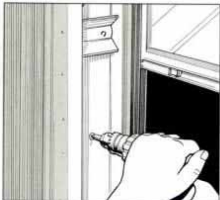
19 A jamb liner with a spring-loaded channel on the left side of the window allows the window to be removed.
