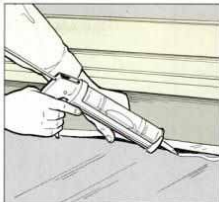
22 Lift flashing slightly and apply a generous bead of silicone or other exterior caulk under the flashing.
