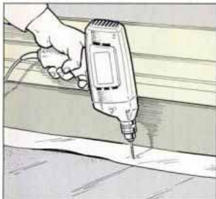
21 Drill through the flashing into the sleeve's top with a \frac{3}{16} -in.-dia. drill. Space holes about 4 in. apart.
