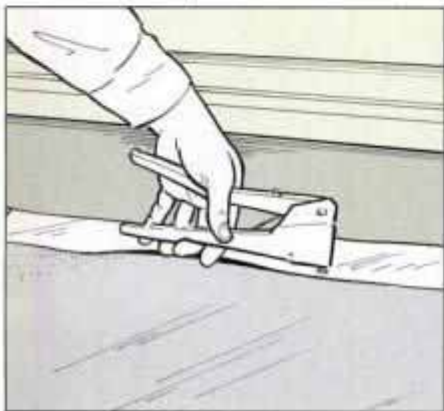
23 Rivet the flashing to the air-conditioner sleeve. Smooth the caulk that is squeezed from under the flashing.
