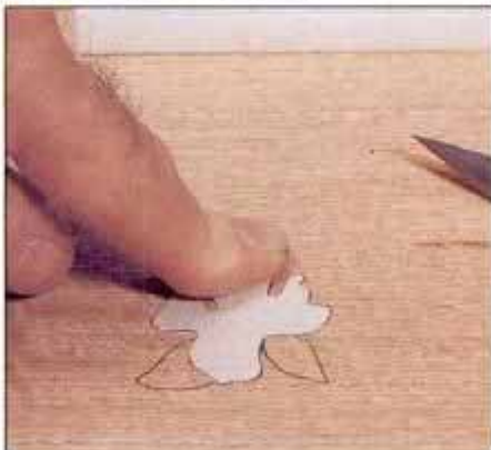
10 Return the cutout piece to the window, press it flush with finger pressure. Then apply tape on the other side.
