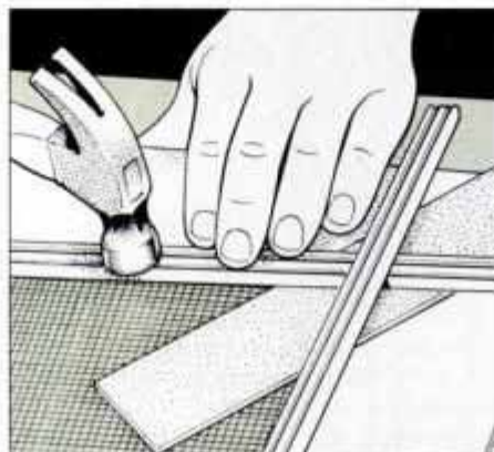
15 Nail screen molding in place, but leave it overlong at the corners. Place cardboard under molding as shown.
