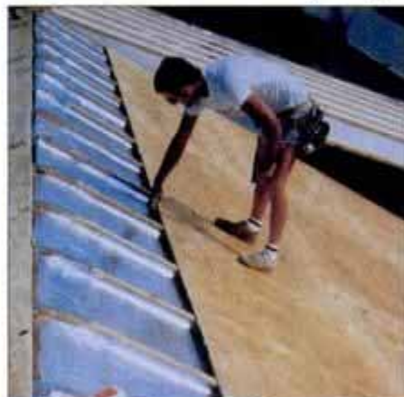
To achieve R-50 in the roof, foam panels are placed between the rafters and covered with foil. Then plywood is installed.
