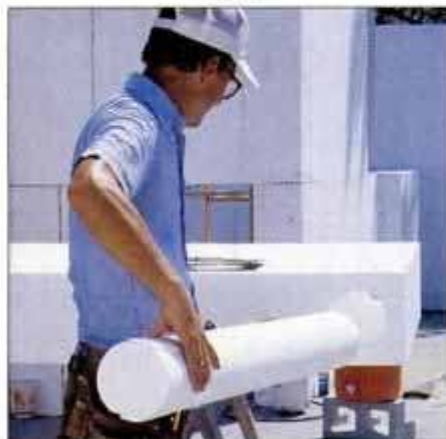
The foam panels are cut to create the hollow post (shown above) and beam cavities that will be filled with concrete later.
