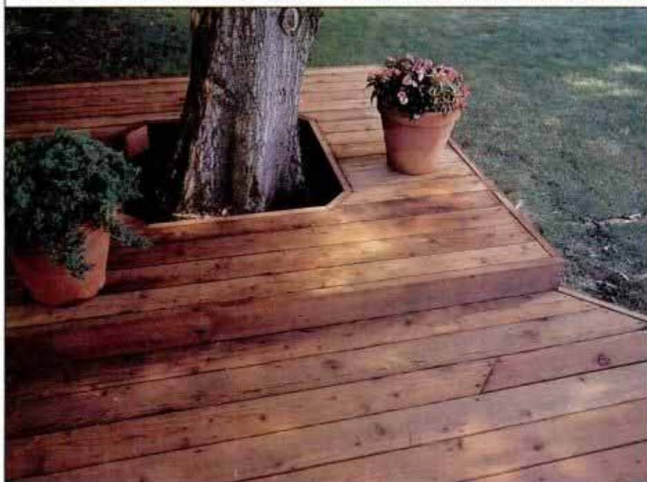
To accommodate a tree next to the main deck, we added a raised section that surrounds the trunk. The inner edge rests on the deck, and the outer edge is supported by posts.
