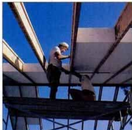
Once the walls are raised and filled with concrete, the roof framing is a fairly typical use of engineered beams and rafters.
