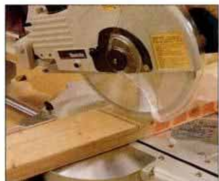
4 Make a partial test cut. Then, shift the stock and retest cut location. Continue test cuts until stock is positioned accurately.
