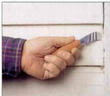
5 To remove cracked caulk from siding joints, use a carpet knife to slice it from both sides. Then scrape out the waste.
