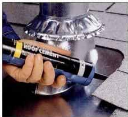
2 Where shingles overlap the flashing, lift up the shingles, apply cement underneath and then press them back into place.
