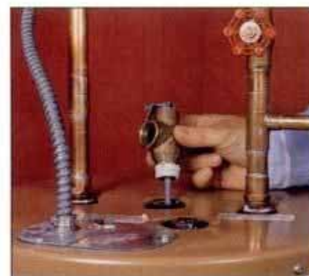
12 If you must replace the relief valve, get a replacement that's properly rated, and install it securely in the top of the tank.
