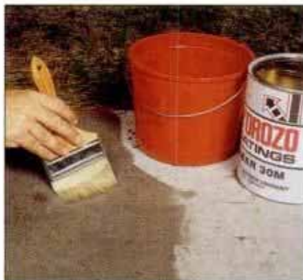
7 To seal driveway surface, it's best to apply a light coat of sealant with a brush instead of using a roller or spray gun.
