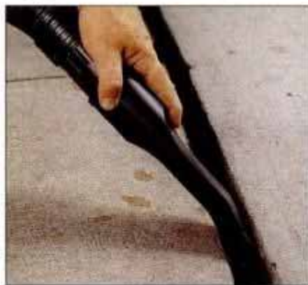
4 Once the major debris is removed from a joint, vacuum out the smaller particles. The joint should be as clean as possible.
