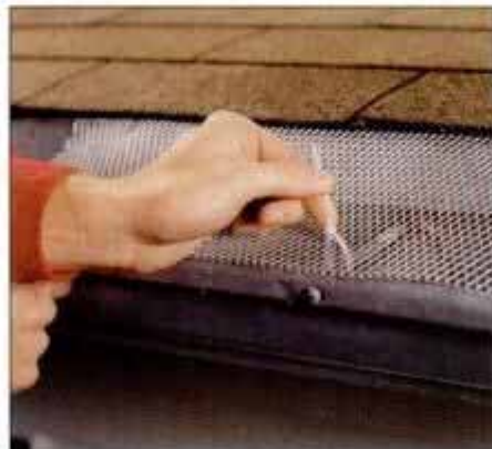
6 To secure the screening, attach it to the gutter brackets using wire or plastic electrical ties like the one shown.
