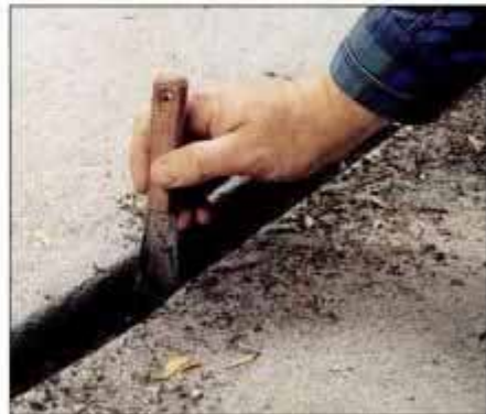
3 To properly seal an expansion joint, first remove all the debris from the joint using a putty knife or cold chisel.
