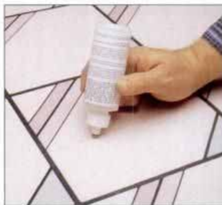
14 Once the mastic is dry, finish the repair by applying seam sealer. Just draw the tip of the applicator over the joint.
