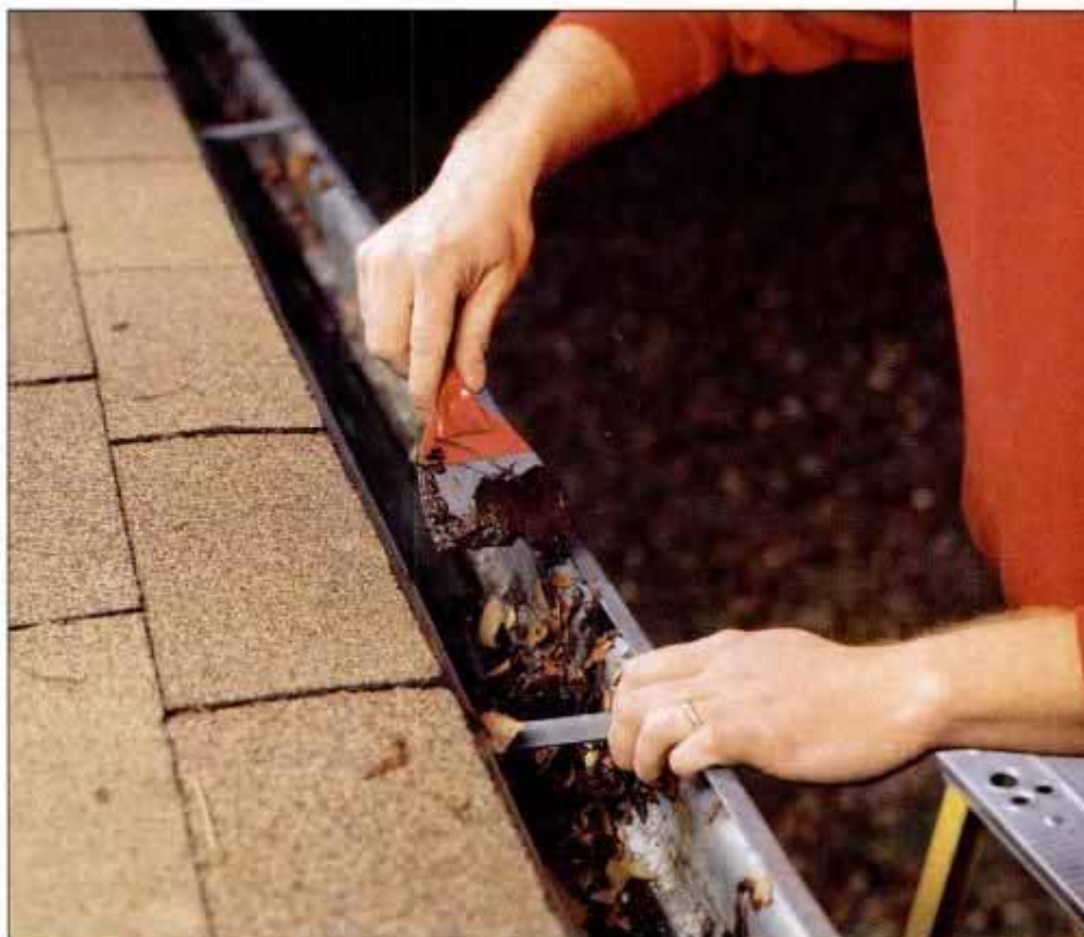
1 Use a narrow drywall or putty knife to remove old leaves and pine needles from gutters. Just scrape the bottom of the gutter clean so water will run freely.
