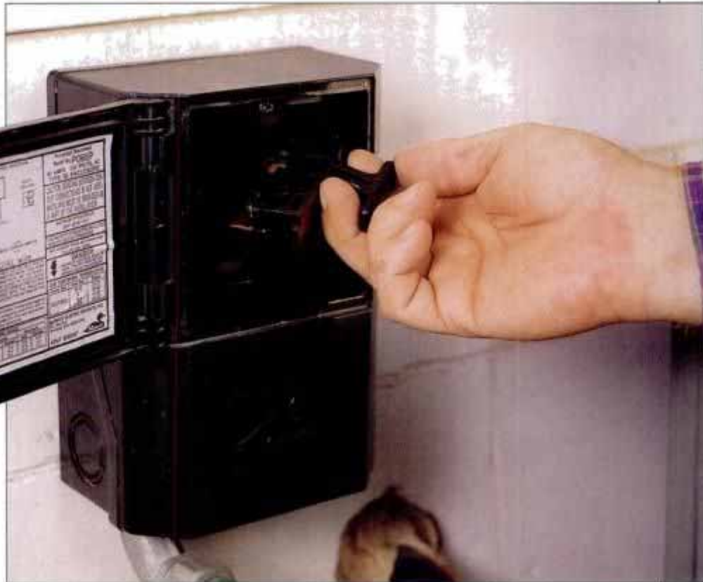
1 Before working on any central air-conditioning system, be sure to shut off the power at the compressor's main disconnect switch or at the house breaker panel.
