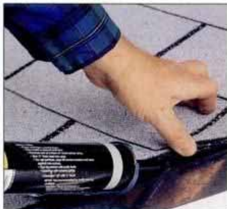
3 If you find a leak where your shingles meet a valley, force roofing compound under the shingles to achieve the best seal.
