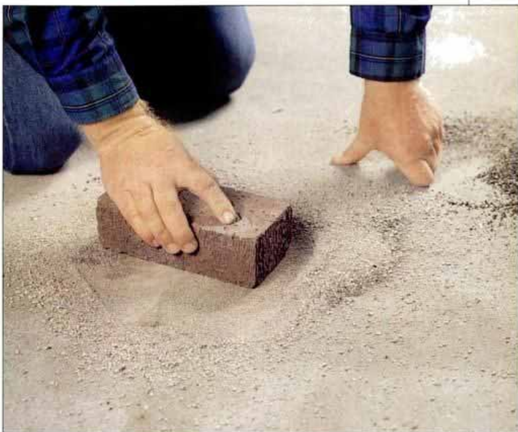
1 To remove an oil-spill stain from a concrete drive, just sprinkle the area with cat litter and rub the surface with a soft brick. Then sweep the area clean.
