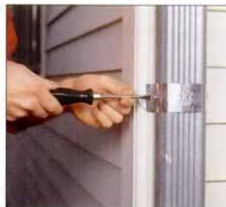
9 Secure all downspouts to the house with brackets. Attach the brackets to the spouts using sheetmetal screws or rivets.
