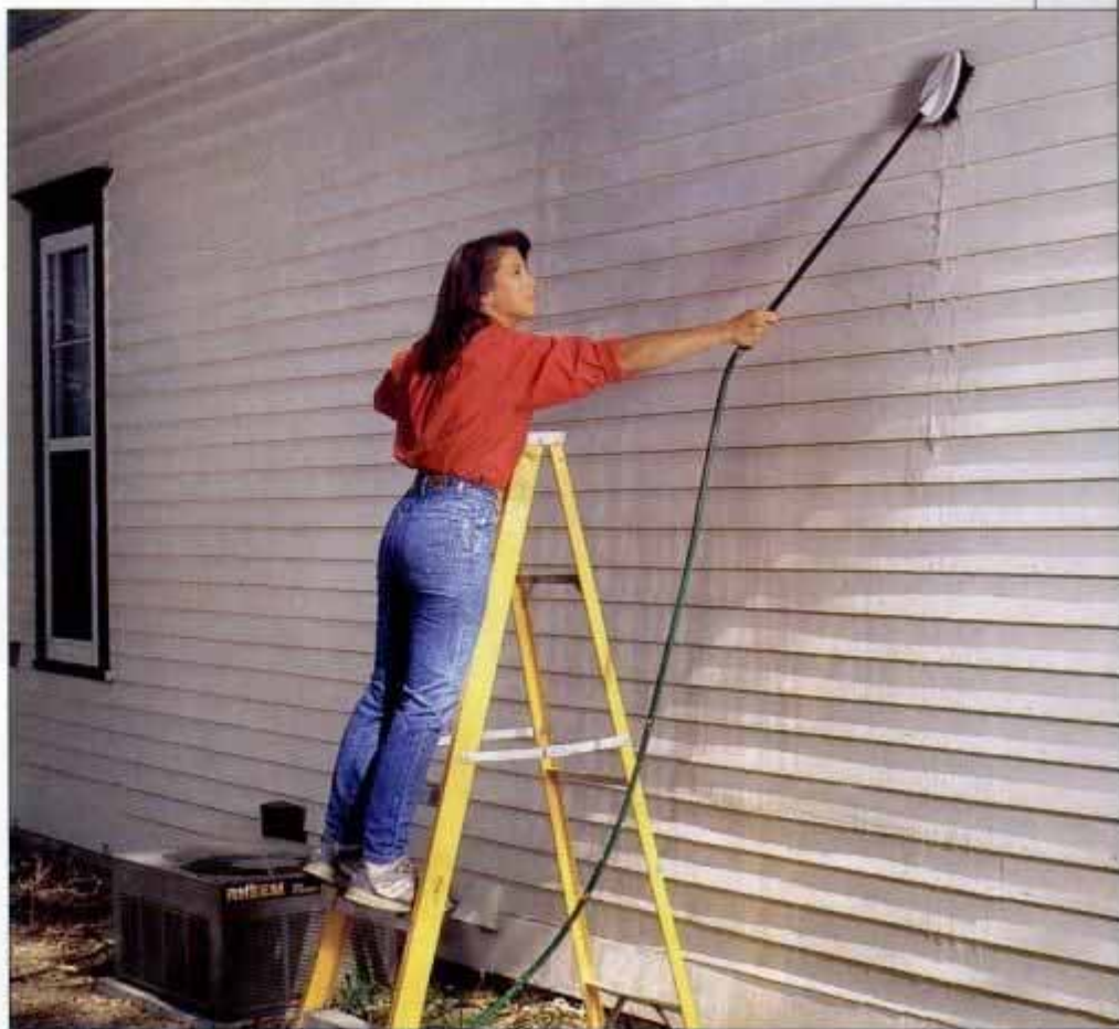
1 To clean your siding, use an inexpensive automotive hose-end brush. Work from the top to the bottom of the wall, washing with a mild detergent and then rinsing clean.
