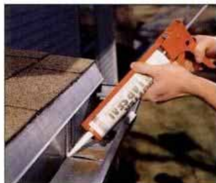
3 Seal gutter joints with a special lap sealant available in caulk tubes. Make sure the gutter is dry before applying.
