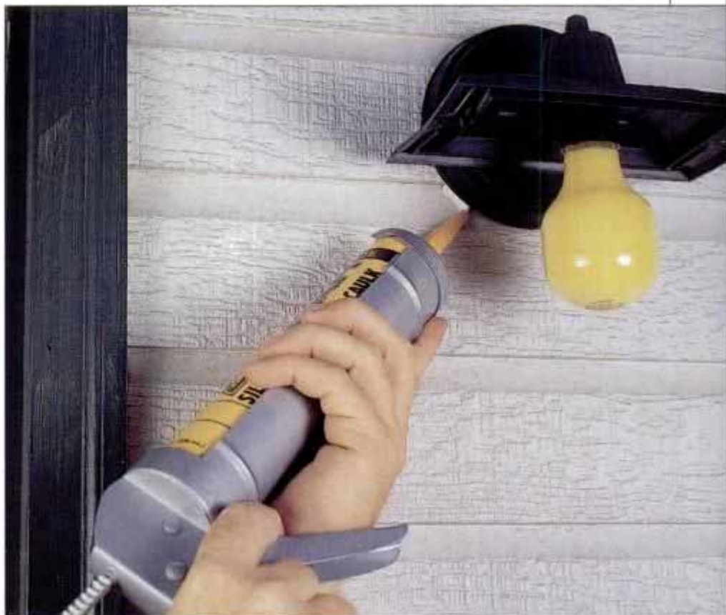
1 Exterior light fixtures, especially those that are mounted on lapped siding, leak like sieves. The voids under the fixture plate can be filled with shim or a neat bead of caulk.
