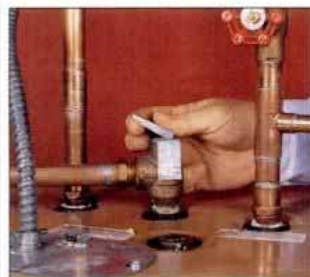
11 Test the relief valve on your water heater by lifting up the test lever and checking that it snaps back completely.
