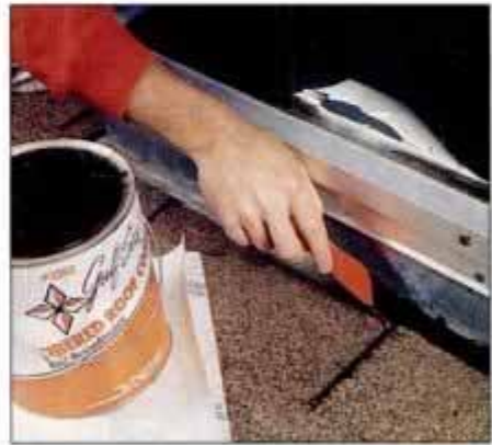
10 Using a putty knife, liberally spread roofing compound across the top of the shingles and against the skylight flashing.
