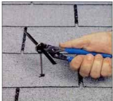
6 TV cable anchors, guyhooks and other roof hardware are best removed if not needed. Most can simply be unthreaded.
