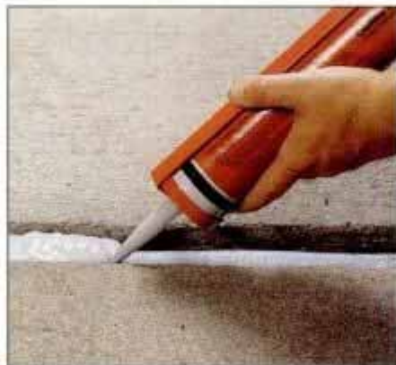
6 Complete filling of expansion joint by covering backing rod with self-leveling urethane caulk, available in tubes.
