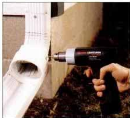
11 A folding downspout extension is a great substitute for a splash block. To attach, first drill pilot holes in both pieces.
