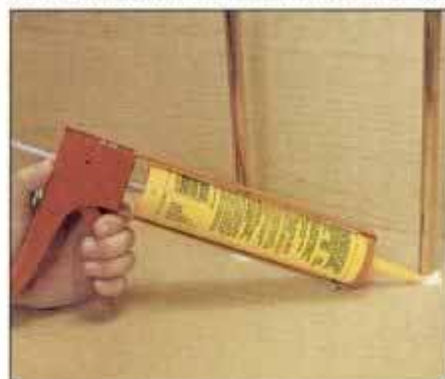
3 Apply caulk to the small spaces around plumbing pipes and electrical lines, particularly in kitchen and bath cabinets.
