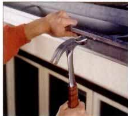
7 To restore the proper slope to a sagging gutter, remove the gutter spike, lift the gutter and re-drive the spike.
