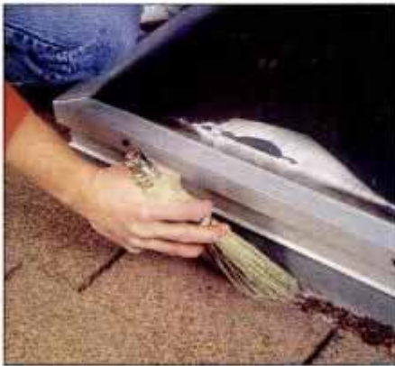
9 To properly seal around a skylight, be sure to remove all debris from around the perimeter. The surface should be clean.
