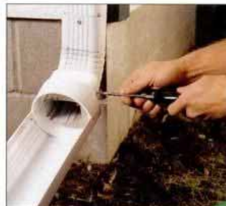
12 Join the extension and downspout with sheetmetal screws. One screw on each side of the downspout is enough.
