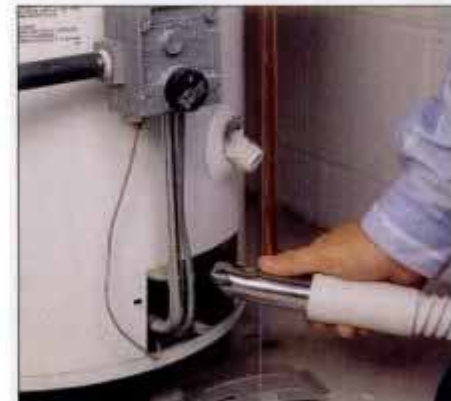
13 To remove rust flakes from the top of a water-heater burner, remove the inspection plate and vacuum out the debris.
