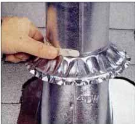
5 Once the storm collar is in place, seal it to the flue with a permanently flexible sealing compound for added protection.
