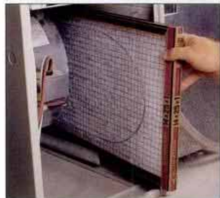
7 Replace the furnace filter every month during peak use periods, and all year-round if the unit heats and air conditions.
