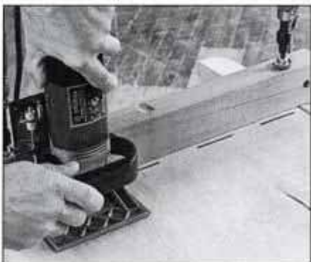
13 Mark the biscuit locations for the shelves on the case sides. Use a straightedge to guide the plate joiner.
