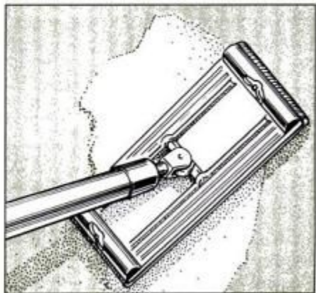
7 Sand the patch level. Use a ceiling sander on a pole if the patch is hard to reach. Apply more compound as necessary.
