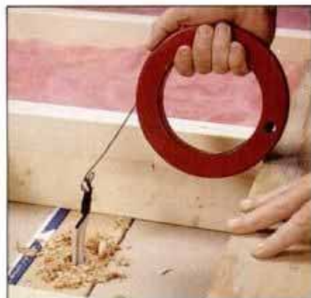
4 Return to the attic and pull the fish tape up to draw the new cable through the hole bored through the top wall plate.
