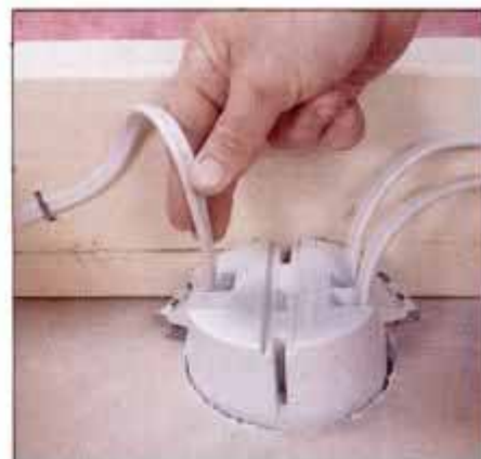
6 Feed new 14/2 cable into an existing fixture box that has power coming to it. This cable will bring power to the new fixture.
