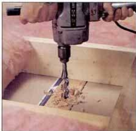
1 Bore 3/4-in. holes through top wall plates to access the stud spaces that correspond to the new switch-box locations.
