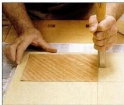
13 Before applying the next veneer section, use a chisel to scrape away glue that has squeezed out along the joint edge.
