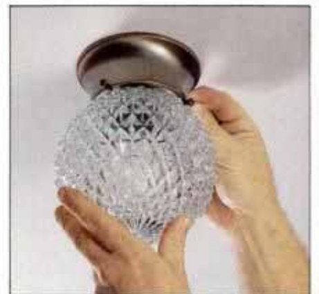
12 When the wiring is done in the new fixture box, install the fixture, an appropriate bulb and fixture globe.
