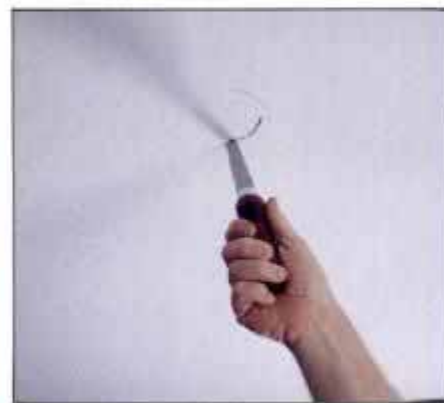
9 Cut 1/4 in. inside the pencil line for the ceiling box opening. This 1/4-in. inset supports the fixture box flange.
