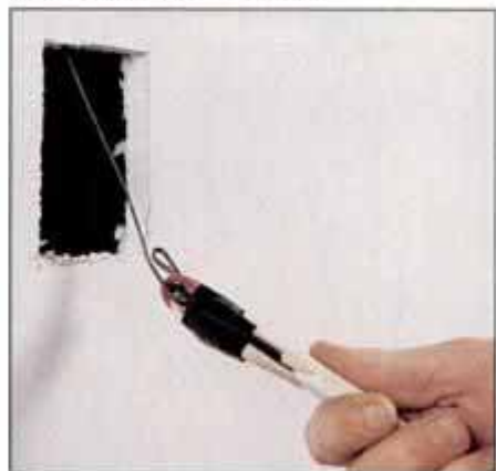
3 Feed a fish tape from the attic to the switch openings and attach the appropriate cable to the tape's hooked end.
