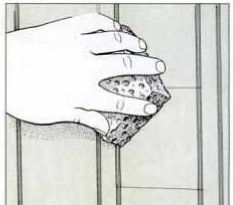
4E Apply glue to patch back and carefully locate in hole. Use a sponge to smooth patch and remove any excess adhesive.
