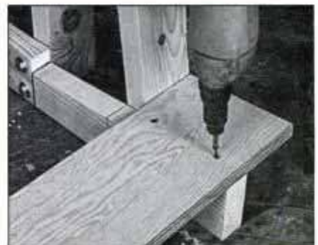
4 After bolting plywood rack uprights to main sections, attach rack base and back support strips with 1 1/2-in. No. 8 screws.
