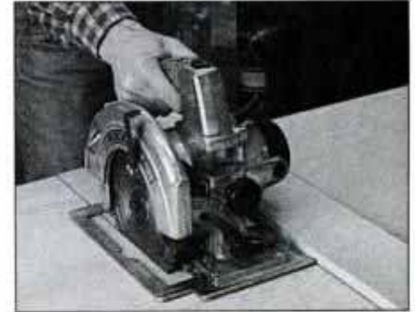
6 Cut plywood for benchtop and shelf to exact size with a circular saw guided by a straightedge clamped to stock.
