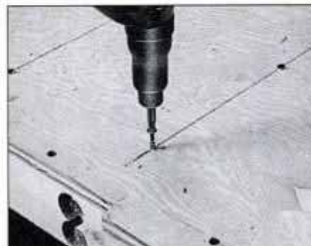
7 Attach top to frame with flathead screws. Countersink screws flush with surface. Note notch in top for vise.
