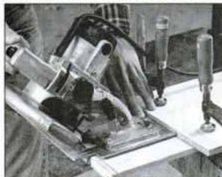
2 Cut the mitered apron ends to length with a circular saw set to 45°. Straightedge clamped to stock guides cut.
