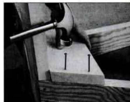
6 Use glue and nails to secure braces to inside edges of legs. Top and bottom brace edges are beveled with hand plane.
