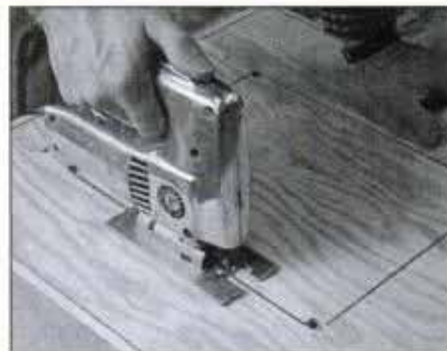
4 After installing plywood top with 6d finishing nails, bore 1/2-in. holes at cutout corners, and finish cutout with sabre saw.
