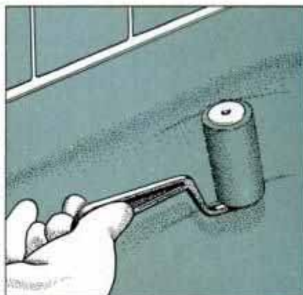
2C Mix the epoxy finish according to manufacturer's instructions. Use a brush and rollers supplied in the kit to apply epoxy.
