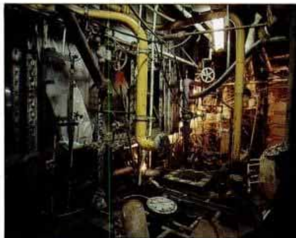
Welder toils deep amid the tangled wires and pipes of the engine room.
