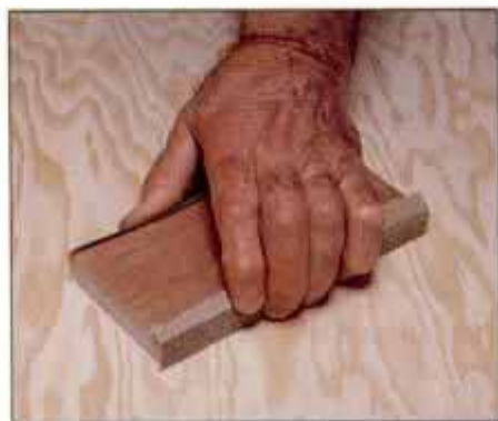
16 Use a large, rigid sanding block on fir plywood. Block spans softer areas for a more uniform and flat surface.
