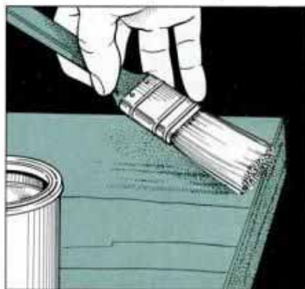
1D Carefully apply a matching stain to the repaired area so it blends with the rest of the door. Then apply varnish to area.
