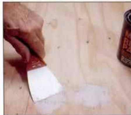
19 Use patching compound to repair defects in plywood that will be painted. Seal with shellac after compound dries.
