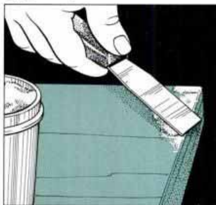
1C After removing clamp, use a putty knife to spread latex patching compound. Avoid spreading beyond damaged area.
