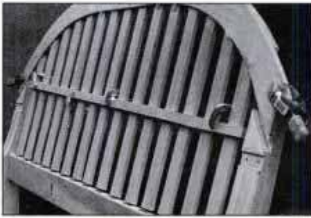
22 Raise arched rail with slats taped and clamped to it. Brush glue into slat mortises, and lower slats into position.
