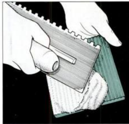
9 To ensure a good bond, spread a thin coat of mortar on tile's ridged back before applying it. Use the trowel's flat face.
