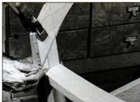
14 Dry assemble the bench with the arched rail clamped in place. Lay armrest on front leg and trace position on rear leg.
