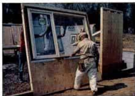
Panelized construction: Once the foundation is complete, the prefabricated walls are brought to the site and erected.
