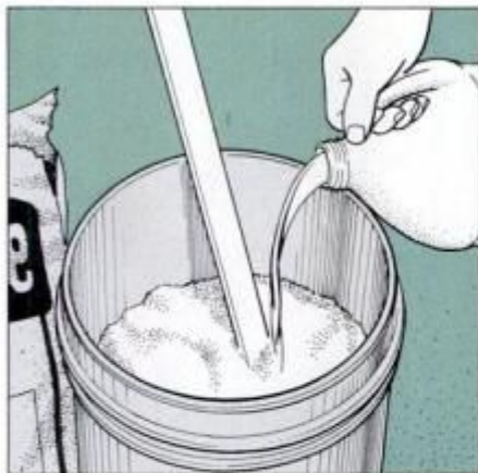
7 Mix an acrylic additive into the dry-set mortar. This increases the mortar's bond strength and its flexibility.
