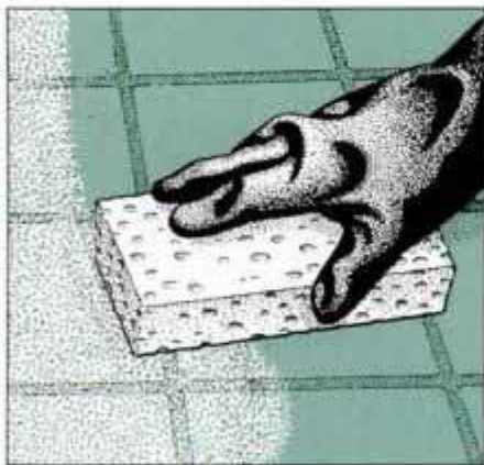
19 Use a damp sponge to remove excess grout from tiles. Rinse sponge frequently in clean water. Wear rubber gloves.
