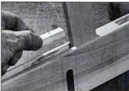
18 Using a dummy slat for spacing, glue and nail spacer blocks in the bottom rail groove. Blocks negate need for mortising.
