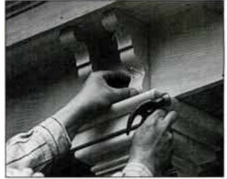
27 Install brackets in pairs over post centers. Then, space additional pairs evenly in between posts. Secure with finish nails.
