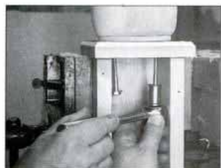
39 Attach each post to a base with two 3-in. lagscrews and washers. Leave off last side until assembly is attached to steps.
