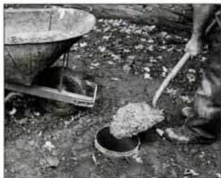
1 Use 10-in.-dia. cardboard concrete forms to pour footings below frost line. Premixed bags of concrete can be mixed by hand.
