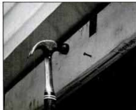
22 Nail notched 2 × 6 rafter ledger to house wall after removing siding. Note aluminum flashing bent up over ledger.
