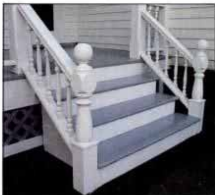
Box-type step construction matches original front porch, as does turned lower newel posts and square upper posts.
