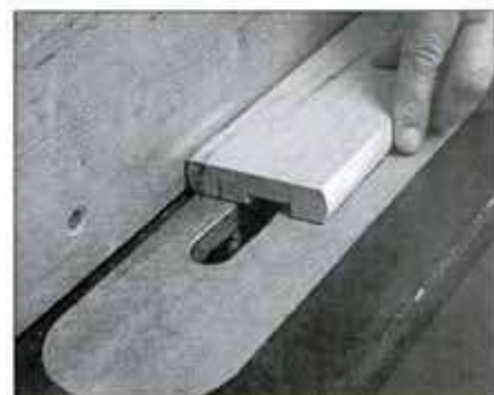
33 Round edges of top-rail bottom section with hand plane. Then, use dado blade in table saw to form baluster channel.
