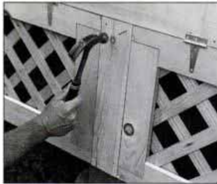
29 Install lattice frames with T hinges (except behind steps). Finish porch floor trim by nailing post trim in between frames.
