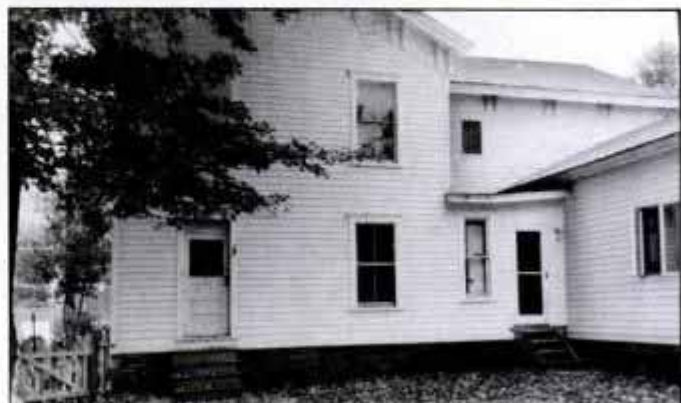
The site before construction shows an extension on the right that abuts a bland expanse of wall. Proportions of the new porch are determined by existing rooflines and door and window heights.
