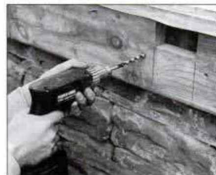
5 After tack-nailing ledgers in place, check that they're level and bore holes for installing the 3/8 x 4-in. lagscrews.
