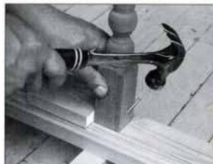
35 Use tapered 2 × 4 wedge under lower rail for support when nailing balusters. Spacer block holds baluster at correct spot.
