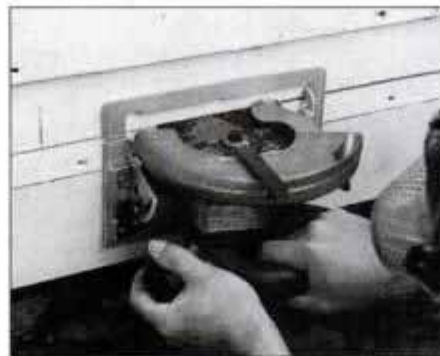
2 After striking chalkline 1/2 in. above floor level, remove clapboard with a circular saw set to cut only through siding.
