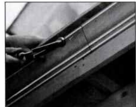
24 When roof decking is done, nail crown molding in corner between deck and fascia. Miter joints between pieces.
