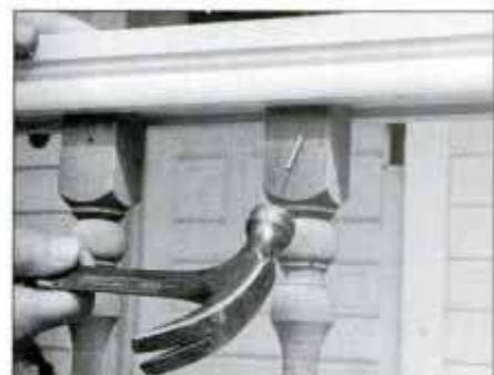
36 Plumb each baluster with a level and toenail baluster to top rail. Set all nails and fill with caulk after priming.
