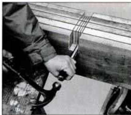
8 Cut notches in the crossbeam pieces by sandwiching them together, cutting saw kerfs and removing waste with chisel.
