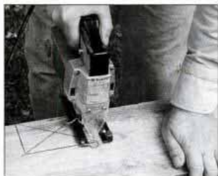
4 After cutting ledgers to length, use a sabre saw to cut the 2 1/2 x 4 1/2-in. ledger notches at crossbeam locations.
