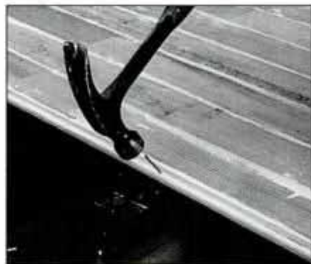
12 Nail 1 x 4 tongue-and-groove flooring to framing. Priming bottom faces and edges increases the life of the floor.
