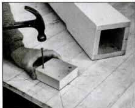
19 Lay out 6 × 6 post centers on floor, and nail 1 1/2-in.-thick post block to floor. Then, install posts, plumb and brace.
