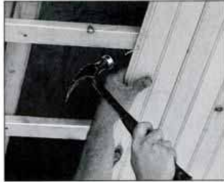
26 After 2 x 4 crossies and 1 x 3 furring strips are in place, secure 1 x 5 beaded tongue-and-groove ceiling with finish nails.
