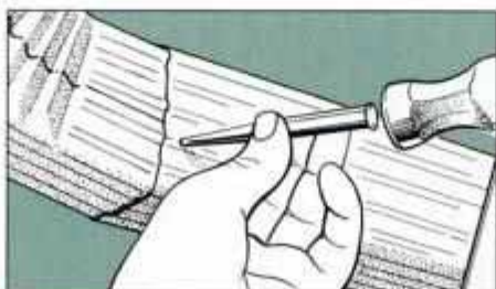
4A Use a metal punch to make a small dent over where you want to drill. Dent holds drill bit as it bites into metal.
