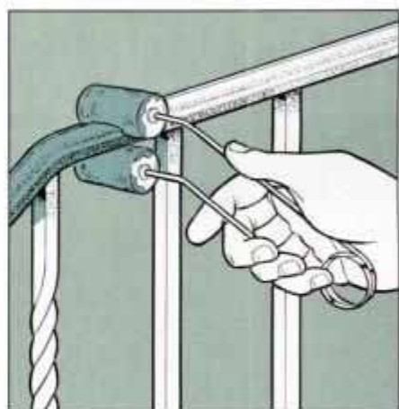
Use a special roller, like the one shown, or an aerosol spray can to paint the ironwork. A flat-black finish is the traditional look.
