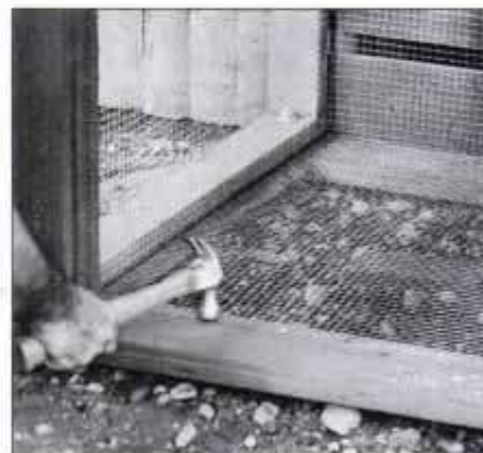
21 Situate the bin on level ground and place a brick at the center of each bin to support mesh. Nail in the bottom mesh.
