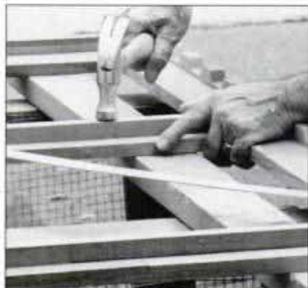
19 Vertical redwood molding is installed on the frame so it aligns precisely with ridges on corrugated molding.
