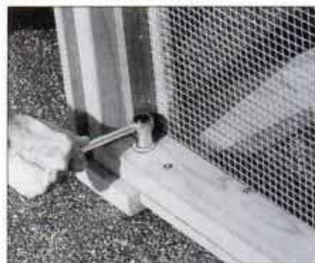
10 Bolt end frames to baseboards after mesh is installed. On end frames, bolts are positioned to clear nailers.
