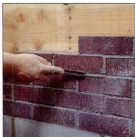
7 Once the mortar in the joint begins to set, strike each joint with a jointer to form a smooth, compressed seam.
