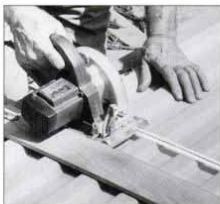
17 Support the panels on corrugated molding. Mark a cutline with tape and run the saw's shoe against a fence.
