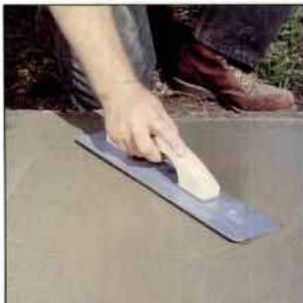
1 After screeding the concrete level with the form, use a hand float to smooth the slab and pull cement to the surface.
