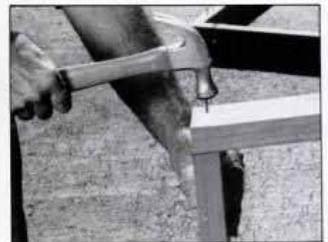
2 Each frame section is made up of four pieces nailed together and marked with chalk to indicate placement.
