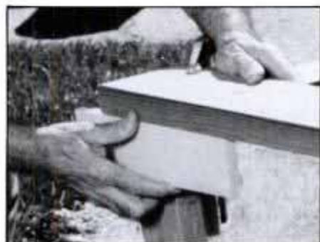
3 With frame inverted, position the baseboards using a scrap block at edge of frame to gauge 1/4-in. overhang.
