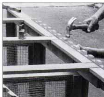
18 Nail the corrugated redwood molding through alternate valleys. Molding is sold with the corrugated panels.
