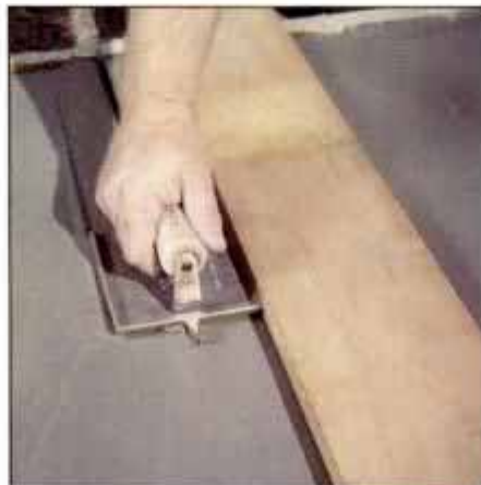
3 Use a groover to cut control joints in sidewalks, drives and outdoor slabs. It should penetrate one-quarter of thickness.
