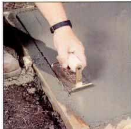
2 When the surface has been floated, compact and round the slab perimeter with an edger. Follow the inside of the form.
