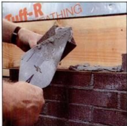
5 Use mason's trowel to first spread mortar along preceding course. Then butter end of the next brick and set in place.
