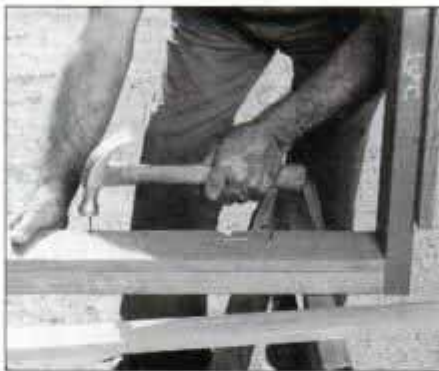
6 Remove baseboards from the frame and attach the front mesh nailers to each frame. Again, use galvanized nails.
