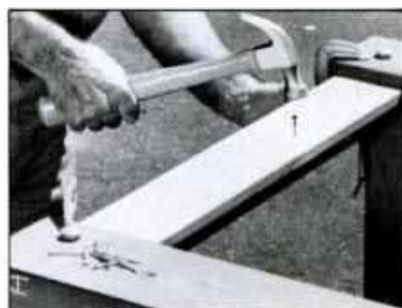
5 With the frame inverted, attach the mesh nailers to the bottom of each frame using 6d galvanized common nails.
