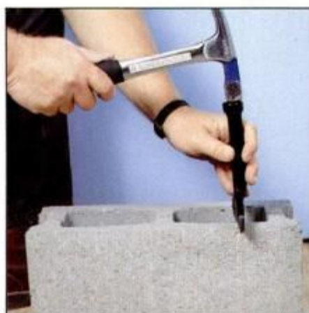
8 To cut a concrete block, tap the chisel lightly in a line completely around the block until the two halves fall apart.
