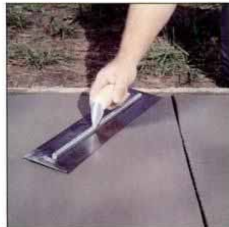
4 Finish by sweeping a trowel in half circles across slab. Hold the trowel nearly level and use two passes for a smooth surface.
