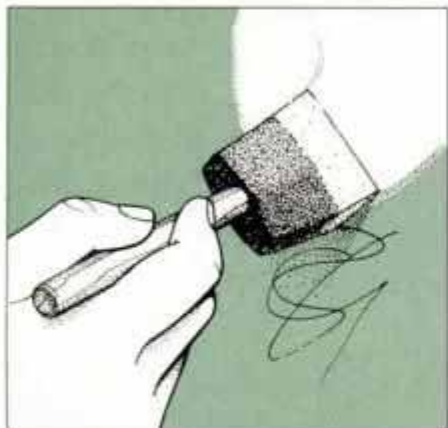
9 Stains bleed through latex paint, so hide them with shellac-based primer. Apply the primer with a foam brush.
