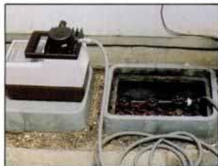
3 Set at 100 psi, compressor made short work out of the annual chore of blowing water from underground sprinkler lines.
