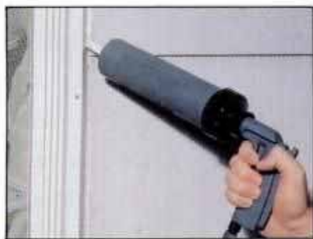
6 Set at 10 psi, the compressor steadily pushed a smooth bead of exterior latex caulk. The caulk gun proved easy to use.
