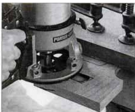
11 Clamp base pieces to bench and run router against a fence clamped to base. Finish dadoes by chiseling them square.
