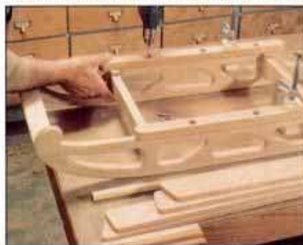
10 Bore post holes in lower rails, and clamp rails to runners. Bore pilot holes for screws that attach rails to runners.
