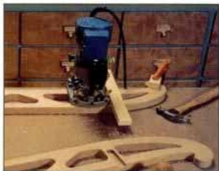
4 Using a router, cut the stopped dados in the runners that house the crossmembers. Guide cut with a scrap block.
