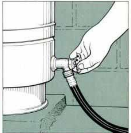
6 If you have a water well, first open all faucets and flush all toilets to drain most of water, then drain pressure tank with hose.
