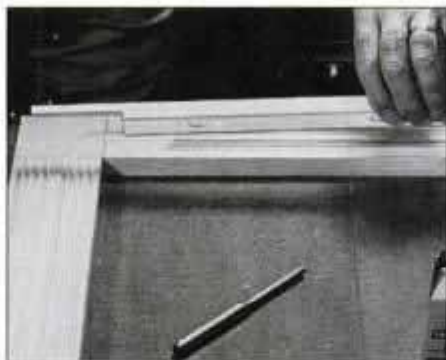
9 First attach the upper and lower rail trim with glue and nails. Apply glue sparingly to the notched end of trim pieces.
