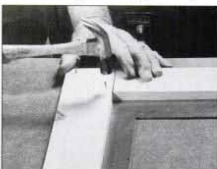
6 Butt a framing square into the frame corners. Apply glue to the joints, and drive in \frac{1}{8} -in. nails from back of joints.
