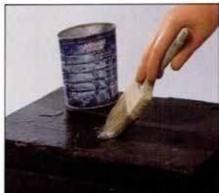
1 Apply stripper with brush in single strokes—avoid brushing back and forth. Work on horizontal surfaces if possible.
