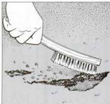
4 To prepare small holes for filling with patching compound, clean out crumbling pavement and dirt using a stiff wire brush.
