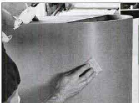
27 Sand primer with 220-grit sandpaper. Note that glue line between half round and pedestal disappears under primer.
