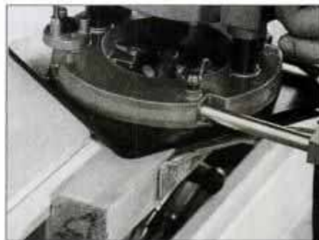
4 Use a \frac{1}{4} -in.-dia. straight bit in the router with a fence guide to cut rabbet on top and back edge of the pedestal panel.
