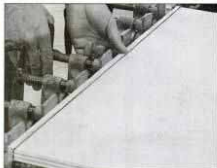
1 Clamp the maple edge bands to plywood panel edges. Note that edge bands are clamped only to a panel's front edge.
