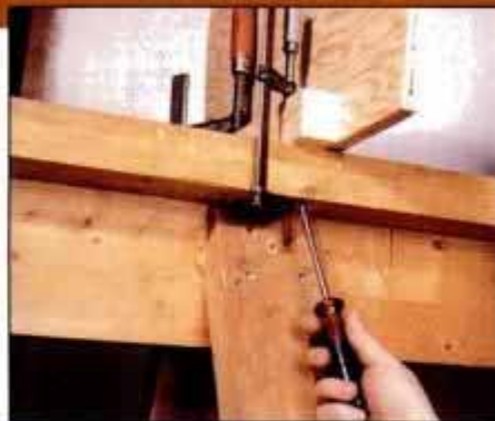
3 When each mold is plumb and square, screw to strongback from below. This allows hull to be removed later.
