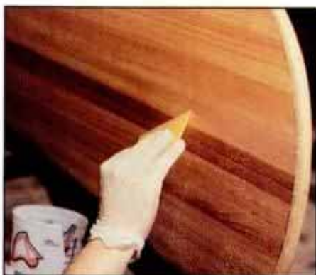
25 After the hull is covered with epoxy, use a squeegee held at an angle to remove excess. Wipe waste in plastic container.
