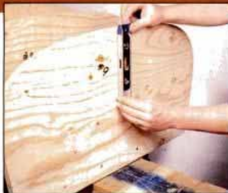
2 Use a level held against the mold centerline to check for plumb. Place shims underneath 2x2 cleat to adjust mold.
