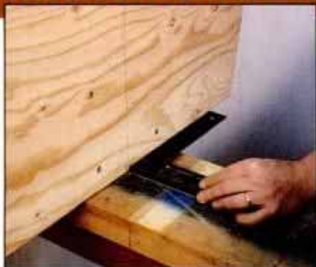
1 Clamp all molds square with centerline. Place every station mold except center mold on midships side of station line.
