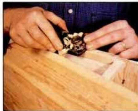
13 As the planking nears the flat run of the stem, bevel the stem to accept the strips and align with first cross-sectional mold.
