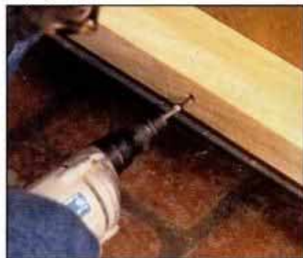
1 To modify cabinet space to receive built-in oven, glue and screw 3-in.-wide wood cleats to cabinet sides to support oven.
