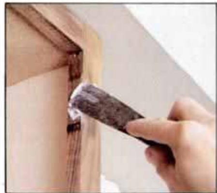
6 If you plan to paint the cabinets, fill all holes, nicks and scratches with wood filler. Push filler in place with putty knife.
