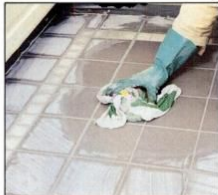
11 Once grout has set up, clean surface with damp cloth. Rinse cloth frequently in clean water to get best results.
