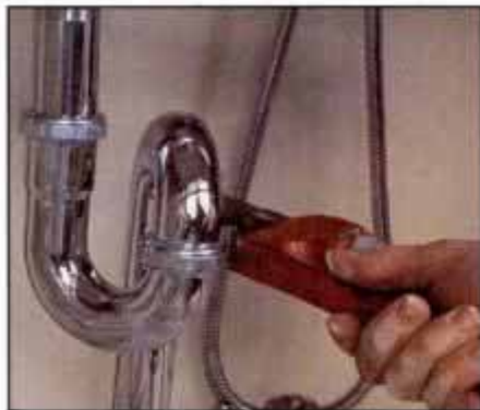
8 Join disposer to waste line with proper tee. Then add trap to waste line and tail-piece. Tighten disposer ring securely.
