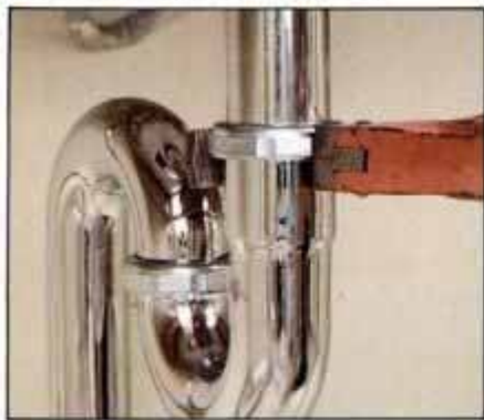
8 To remove sink, loosen nut between tailpiece and trap using pipe wrench or pliers. Pull trap away from tailpiece.
