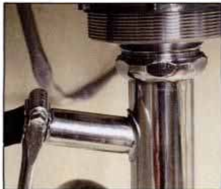
3 To remove dishwasher, begin by loosening clamp that holds drain hose to sink tailpiece or to disposer. Pull off drain hose.
