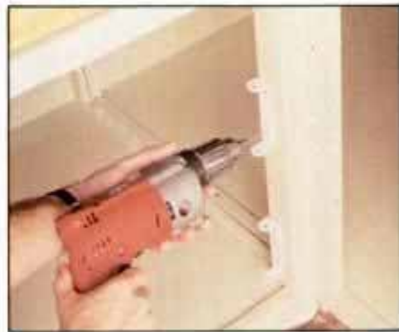
4 Quarter-turn shelves are great for corner cabinets. To install, prebore pilot holes, then screw brackets to edge of face frame.
