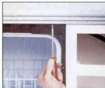
13 Attach upper corners of dishwasher to underside of counter with screws driven up into substrate, not countertop material.
