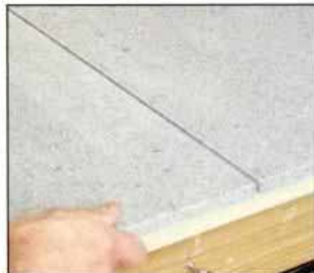
6 Once seam is cut, slide mating sheets onto cabinets and check for fit. If fit is tight, then cut other end of sheet to length.
