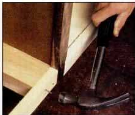
2 Cut bottom rail to match size of existing cabinet rails. Then, attach to oven support cleats with glue and finishing nails.
