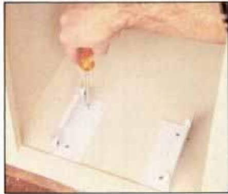
2 Prebore pilot holes, then mount trash holder roller brackets to cabinet floor using screws provided. Tighten screws securely.
