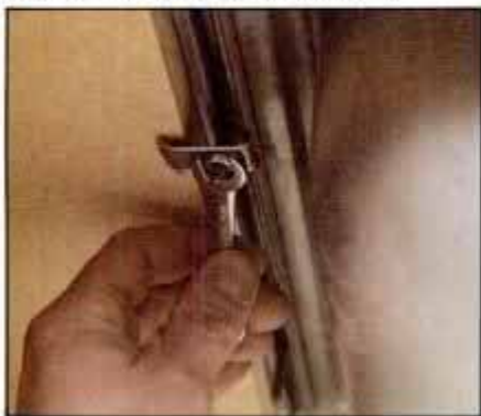
10 Using a wrench, remove sink hold-down clamps that bear on countertop. Run putty knife under sink rim to free up sink.
