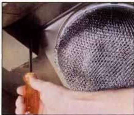
1 To remove range hood, first shut off circuit power. Then, using a screwdriver, remove the hood's junction box cover.
