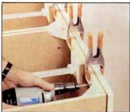
5 Cut \frac{3}{4} -in. plywood back to same size as front face frame. Clamp in place and attach with screws driven through cabinet back.
