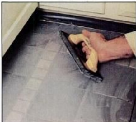
10 Remove excess grout as you work by holding trowel at 45° angle. Less grout left on surface makes cleaning up easier.
