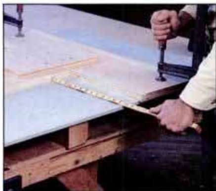
4 For a U-shaped counter, do not make joints at corners. Instead, clamp L-shaped guide to surface and cut returns on ends.
