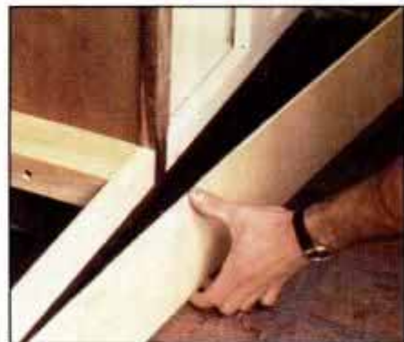
3 Install toe kickboard—made of 1/4-in.-thick plywood—on adjacent cabinets to span oven cabinet opening. Nail in place.
