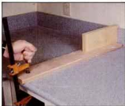
11 Join backsplashes to counter and walls with silicone adhesive. Clamping jig holds pieces until adhesive sets.
