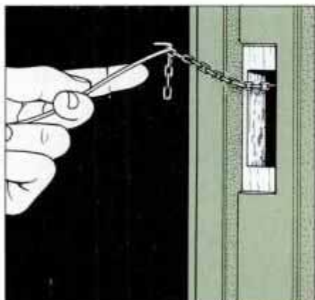
12 Fashion a hook on the end of a hanger wire, then use the wire to retrieve the chain from stud cavity behind the jamb.
