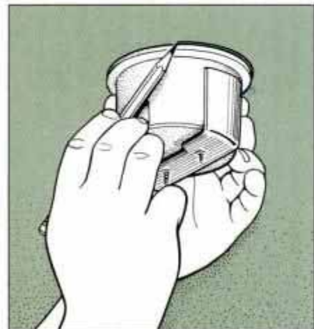
1 Locate a cavity between ceiling joists and hold a cut-in box against the ceiling in this area. Trace around the box perimeter.
