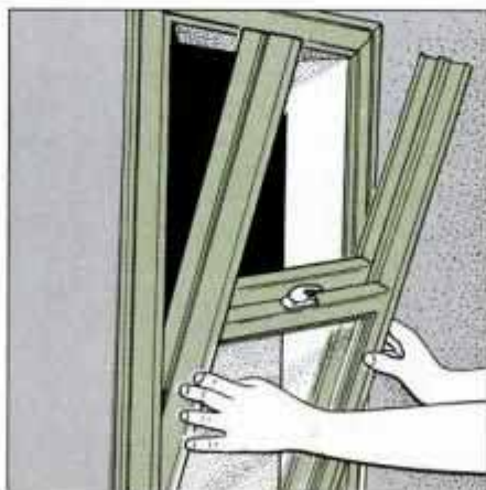
19 Discard window weights, pulleys and parting strips, slide channels and sashes in place, bottom first. Reinstall sash stops.
