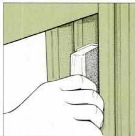
4 To create a smoother sash channel, wrap sandpaper around a wood block and sand the edges of the stops and parting strips.
