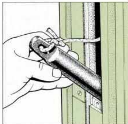
14 Lift weight from opening to replace cord with chain. With some windows, casing trim must be removed to gain access.
