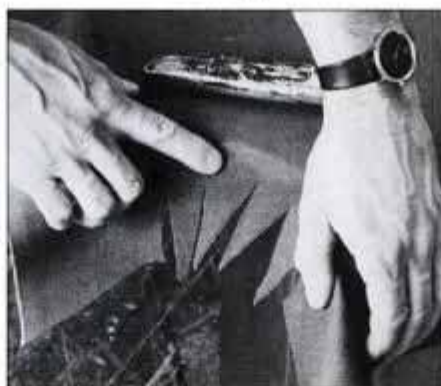
34 Make radius cuts at corner pockets. Stop cuts 1½ in. from slate edge. Pull each triangle tight and staple to frame.
