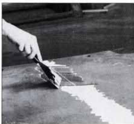
31 Spread plaster of Paris over joints and scrape joints smooth with 6-in. flat knife. Fill the screwholes with plaster.
