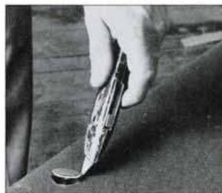
35 Cut away cloth over holes for the rail bolts. Completely remove the cloth to ensure maximum rail bolt adjustment.
