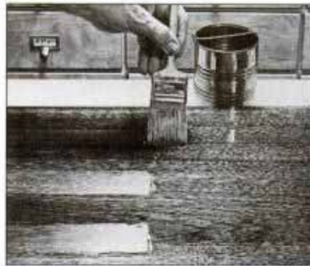
6 Without adding new varnish, brush across grain for even coat. Always use an extralight stroke when leaving edge.
