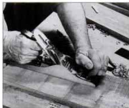
3 Plane the entire surface flat and to guideline marked on one edge. Check frequently with straightedge and winding sticks.
