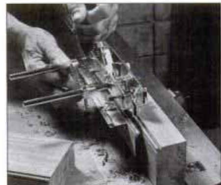
18 Install a 1/4-in. bead cutter in the combination plane and cut a half round from both surfaces for the 3/4-round molding.
