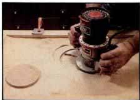
3 Remove template and finish cutting the recess. To ensure support for router, cut away waste moving from front to back.
