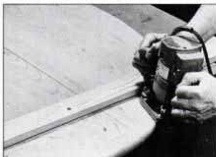
7 Clamp top together with C-clamps and long boards that span joints. Rout edge profile with 1/2-in.-dia. quarter-round bit.
