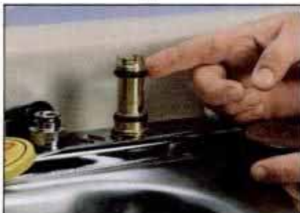
After replacing spout O-rings, lubricate them with heat-proof grease and press the collar over the O-rings and faucet body.
