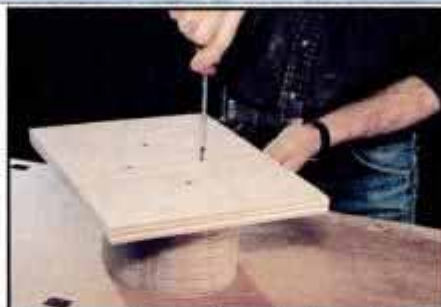
2 Screw a plywood base to the mold bottom to act as a clamping fixture. Cut base 4 in. wider and 8 in. longer than the mold.
