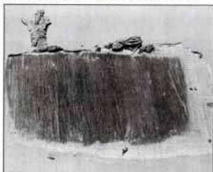
This section of wall paneling had been painted with latex. Stripper not only removed the paint, but also the factory-applied finish.
