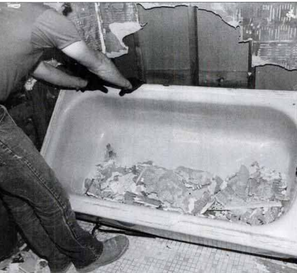
If you want to remove—or relocate—a plumbing fixture, the job requires more than just taking the old fixture out. You must also cap off the old plumbing behind the surface of the wall.
