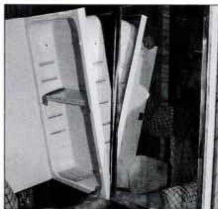
2 Slide first cabinet in place and check for plumb. Screw into framing. Hold second cabinet in place and check for mirror swing.
