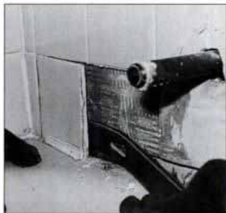
4 Remove tile from around tub using a flat bar. If you plan to keep the tub, be sure to protect it with cardboard or a blanket.
