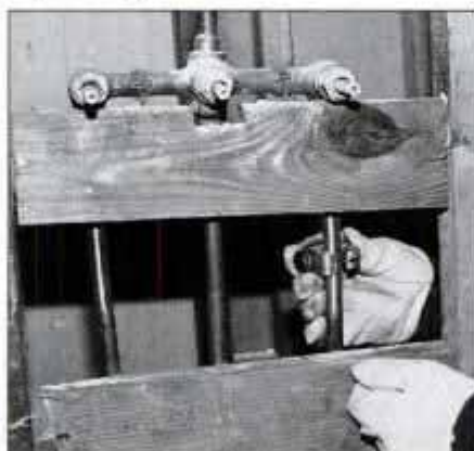
2 Remove the fixture and the wall covering behind it, then cut the rough plumbing with a tubing cutter. Don't use a hacksaw.
