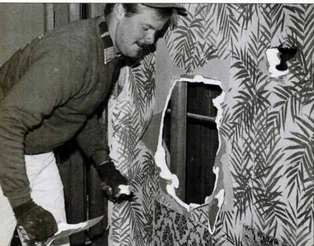
There is more to demolition than simply tearing out everything in the room. A good strategy is required to keep the mess to a minimum and prevent personal injury.
