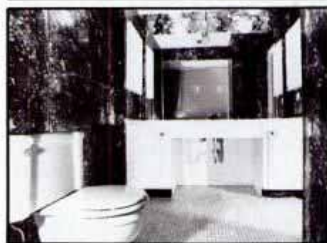
Hi-tech bath (top) was made possible by gutting room (above) and adding new fixtures, flooring and metal laminate to walls.
