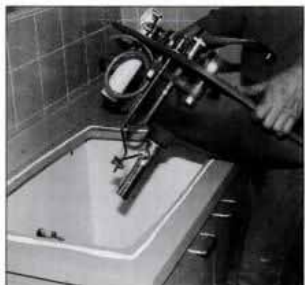
4 Apply silicone caulk around perimeter of sink opening, then lower sink into place. Center in opening and wipe away excess caulk.
