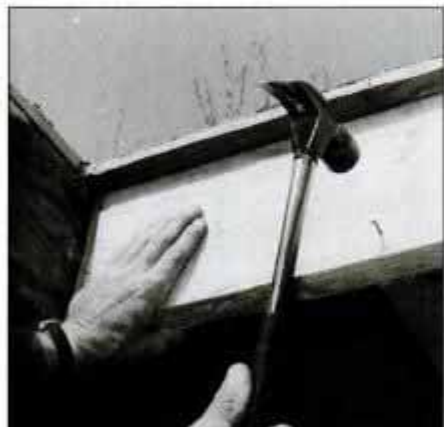
4 Cut rafters that fall in opening, then cut and nail header stock in place. Header transfers weight to the adjacent rafters.
