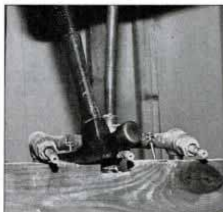
3 Once old supply lines are cut, pry them from the wall and set aside. Frequently, they can be reused, so don't throw them away.
