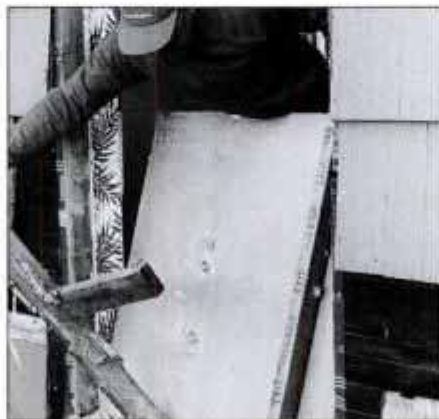
4 Once the siding is removed, pry out cripple studs below window sill and remove any drywall or plaster from inside the room.
