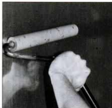
6 Once each panel is in place, carefully roll entire surface with a laminate roller. This ensures the best bond and a smoother surface.
