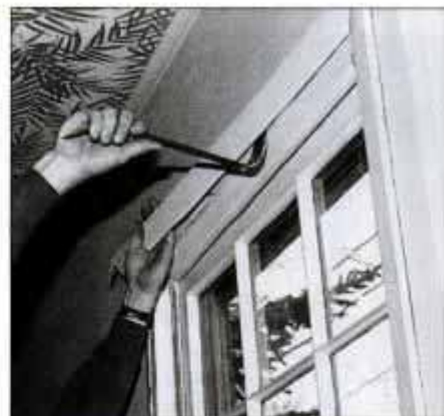
1 Begin by removing the interior casing from your window using a flat bar. Be careful of this trimwork if you plan to reuse it later.
