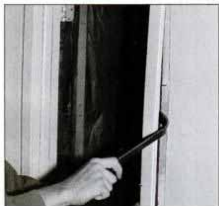
1 First remove all of the casing material from the window and the door jambs. Use a flat bar or crowbar for this job.
