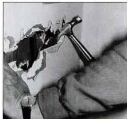
5 Remove drywall or plaster with a straight claw hammer or flat bar. Wear a high-quality dust mask and eye protection at all times.
