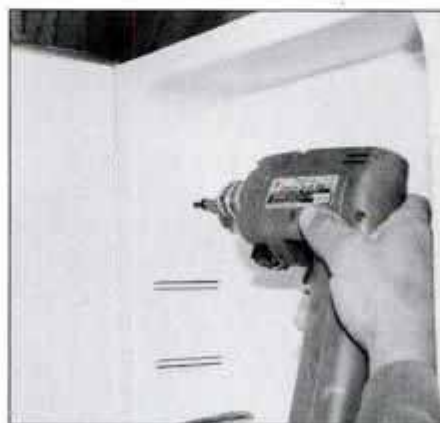
3 Attach all cabinets to framing using drywall screws. Screws allow cabinet to be removed without damage.
