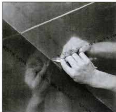
4 Because no room is absolutely square, cut wall panels slightly oversized, then hold in place and scribe to fit the ceiling panels.
