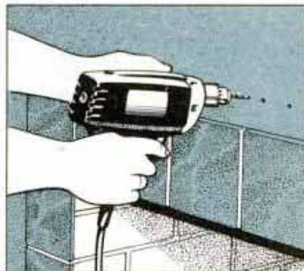
2 After finding the general location of studs by tapping on wall, use a 1/8-in. drill bit and bore holes to find stud centers.
