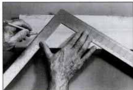
5 Hold square securely and mark plumb cut along edge of square. Mark indicates centerline of ridge board, not cut line.
