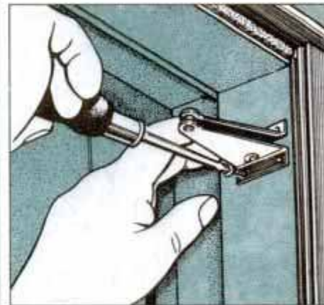
13 Screw the jamb bracket in place, as shown, to support the automatic door closer. Fasten it with four 1 \frac{1}{2} -in. No. 12 screws.
