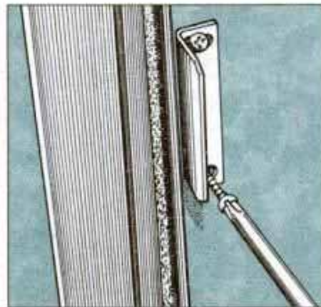
12 A simple L-shaped strike plate is used to engage the latch and hold the door closed. Screw strike plate to door jamb.
