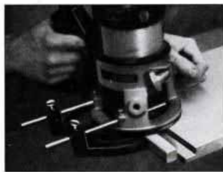
13 Cut long base sides for bed to size, then cut rabbets at the ends using a \frac{3}{4} -in. straight bit and router edge guide.
