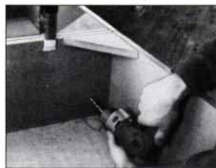
15 Assemble both bases and glue corner blocks in place. Clamp bases together and bore clearance holes for connecting screws.
