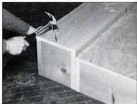
3 After attaching the plywood platform, secure the two long top caps followed by the short top cap. Then attach the 1x12 side trim.
