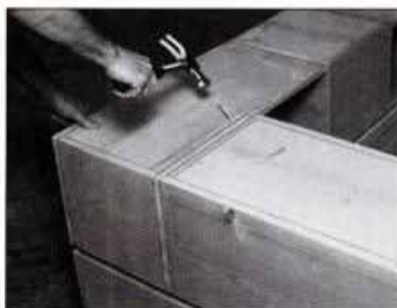
14 With components completed, join the first tier of modules to base with 1 1/4-in. No. 8 fh screws. Toenail modules 3 and 4 at corner.
