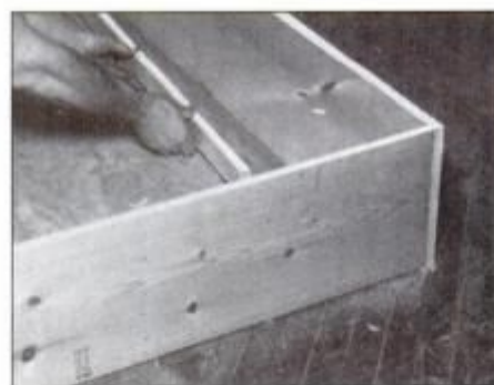
5 Cut the inside trim pieces to size and apply to base frame around the plywood. Plane edges if necessary so they're flush with caps.
