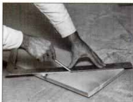
10 To lay out large top spacer miters, align a large steel square so the same number on each leg lines up with edge of stock.
