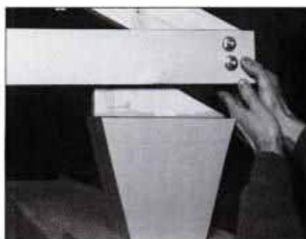
18 Place trusses over keystone supports and secure with 2-in. No. 10 fh screws. Install ridge with 5/16 x 3-in. lagscrews.
