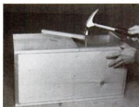
7 Modules 1 and 3 require \frac{3}{4} -in.-sq. strips on side opening edges to bring edges flush with top. Nail with 6d finishing nails.
