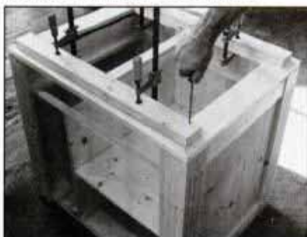
14 Cut the \frac{1}{4} -in.-thick spacer blocking to length and clamp in place. Secure to cap assembly with 2-in. No. 8 fh screws.
