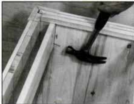
10 Cut drawer guides to size and attach to the corner blocks. Then, install the drawer support strips to the sides, back and front.
