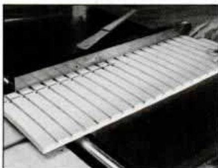
16 Set table saw fence to rip \frac{1}{4} -in.-wide strips of dentil molding. Miter pieces and install with finishing nails and glue.
