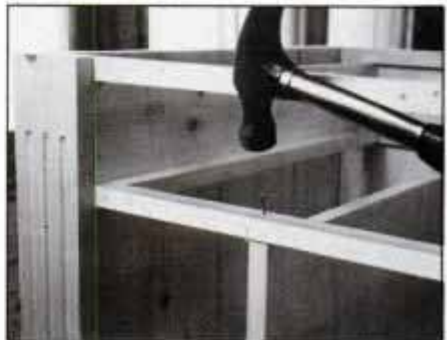
12 Slide partition in and nail up through bottom. Secure top edge by nailing through front and rear drawer supports.
