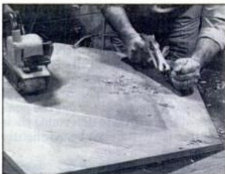
8 Smooth the tabletop surfaces with a belt sander or hand plane for a good connection to rails and a smooth, flat top surface.
