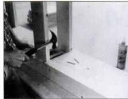
6 Install the bottom shelves so their edges are flush with the base trim. Secure with glue and 8d nails. Set all nails with nailset.
