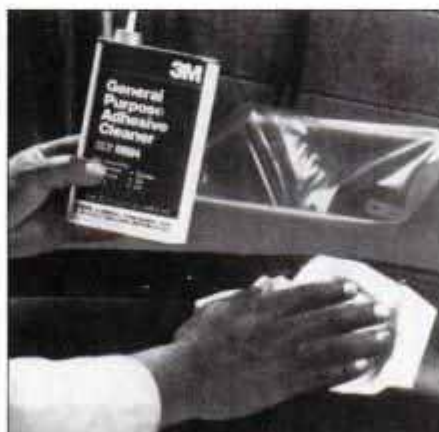
Clean the repair area with a grease, tar and oil solvent. Wipe off any of the excess.
