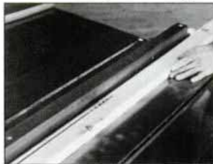
14 After routing both corners to make the half-round profile, rip the shelf trim to \frac{5}{8} in. Top trim is ripped to \frac{3}{4} in. wide.
