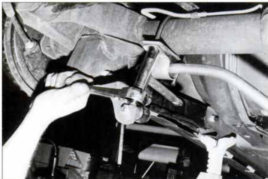
Adding aftermarket antiroll bar should take an hour or so with simple hand tools.
