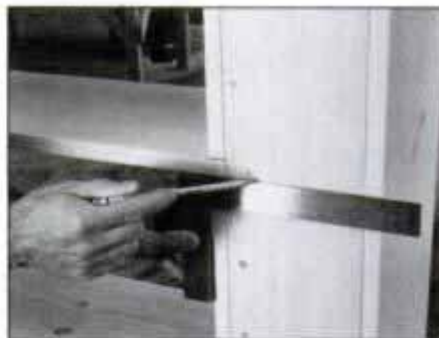
15 Use a square to lay out molding position around end columns and across center column face. Miter trim to length.
