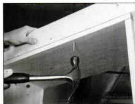
10 After installing the upper trim in the same manner as the base trim, nail up through the top shelf for a tight joint.
