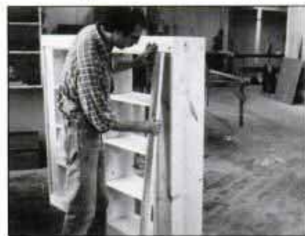
11 Installing end boards leaves a recess for the upright trim. Cut to exact width and length. Nail and glue in place.
