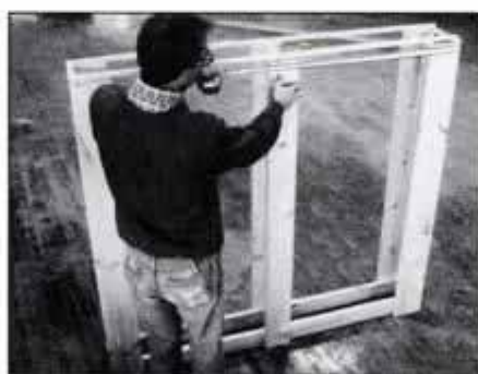
3 Tack temporary strips to the upright tops to ensure consistent spacing. Leave nail heads exposed for easy removal.
