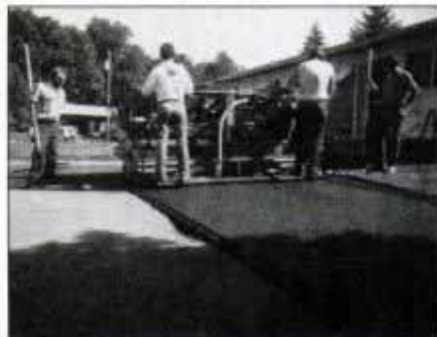
10 As the paver moves along, it lays down a smooth bed of steaming hot asphalt. Two men steer and operate the machine.
