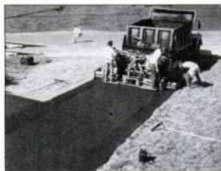
11 The paver, continuously refilled by a dumptruck, never runs out of asphalt. Asphalt bed is 2 in. thick and 10 ft. wide.
