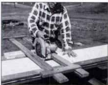
12 Shopmade crosscut guide makes it easy to cut 8-ft.-long siding panels. Place siding under guide, facedown, and cut.
