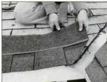
2 When course reaches valley, cut shingle to match old valley line. Keep all nails at least 4 in. back from exposed flashing.
