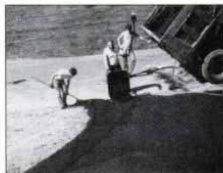
12 The very end of the driveway—where it flairs out to meet the road—is formed by hand. A wheelbarrow transfers asphalt.
