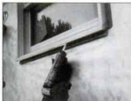
4 Apply caulking to the underside of the window prior to installing the trim board. This helps seal out wind-driven rain water.
