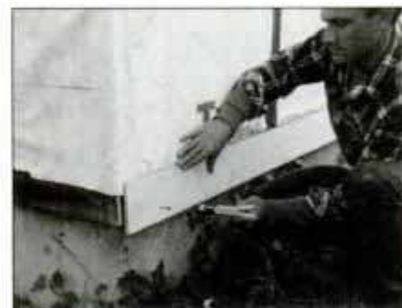
8 Before installing the siding, nail a \frac{1}{2} -in.-thick starter strip along the bottom of the house to build out the first course slightly.
