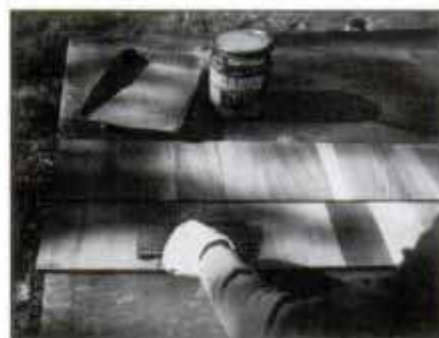
7 Here's a timesaving step: Stain all the siding before installation. A short-nap pad applicator makes staining quick and easy.
