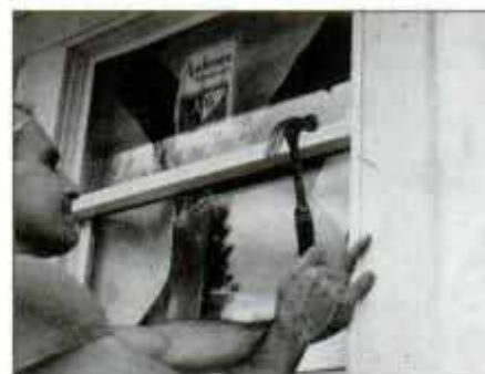
6 Install the vertical pine trim to each side of the window. Fasten the \frac{3}{4} -in.-thick trim with 10d galvanized finishing nails.
