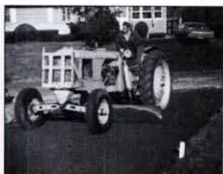
6 A grader smooths the processed stone surface by removing high spots and filling low areas. A 1½-ton roller compacts stone.
