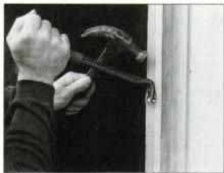
1 Old wood-framed door was nailed through casing. Use cat's paw to pull nails. Remove door and jamb from opening.
