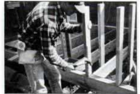
12 Front studs positioned on double 2x8 header must be toenailed in place. Nail studs flush with outside edge of header.
