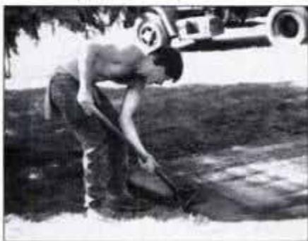
14 The driveway's edge is compacted and beveled slightly with a tamper to prevent it from crumbling under the car's weight.
