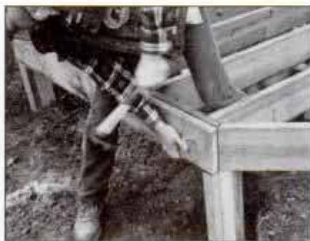
8 After installing all joists, nail a second 2x8 to header. Add 2x4 wood cleats to posts to support the double 2x8 header.
