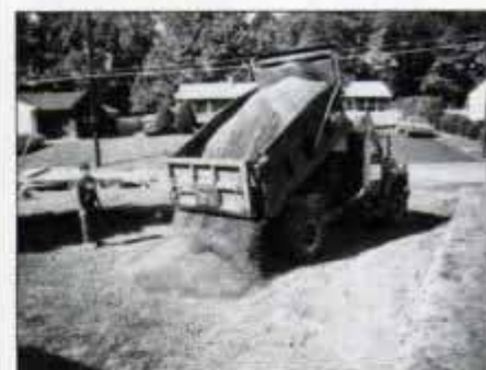
3 Processed stone—a mix of stone and stone dust—is brought in and dumped by truckload to give a stable base for asphalt.
