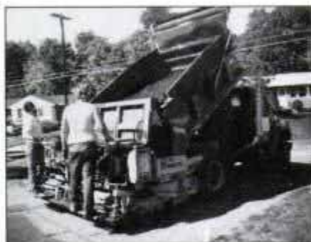
9 The asphalt, picked up fresh that morning, is dumped into the power paver's hopper. The asphalt is approximately 325° F.
