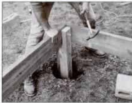
5 Nail 4x4 post to the header joist with 16d galvanized nails. Note how post is notched to form a shoulder to support joist.
