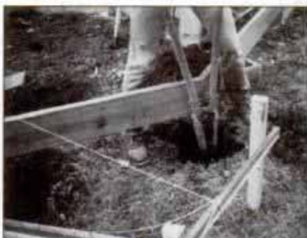
3 A post-hole digger makes quick work of post holes. Dig down about 6 in. below frost line and add 4 in. to 6 in. of fine gravel.
