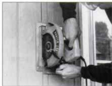
3 Double check your measurements of the rough opening. Use a circular saw to cut through the exterior siding and sheathing.
