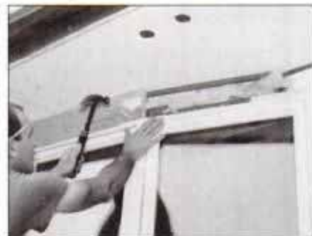
6 Nail exterior trim along top of window. Cleats attached to soffit provide nailing surfaces. Note insulation behind trim.
