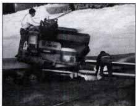
7 With driveway graded, rolled and ready for asphalt, the Power Box—a self-propelled power paver—is driven off trailer.
