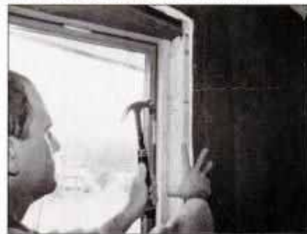
9 Nail a scrap wood block to jack stud on sides of window. This is necessary to provide solid nailing for extension jamba.
