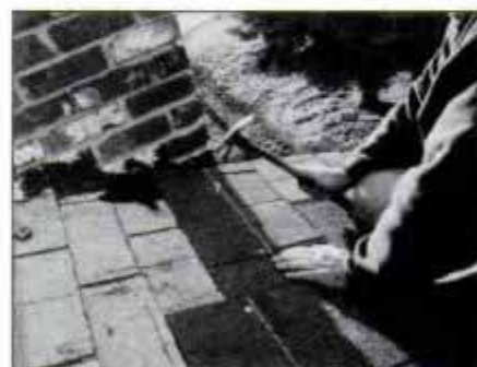
9 Cut and nail next shingle over cement, then continue layering cement and shingles until you are past the chimney or vent.
