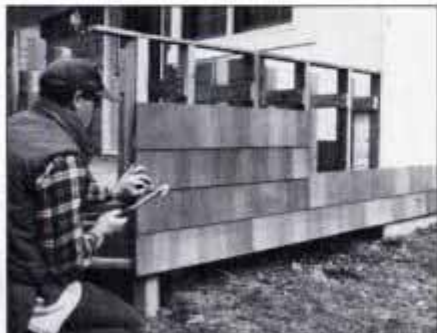
17 Install cedar siding across the deck walls and onto the house. Cut the siding panels so that all butt joints fall on a stud.
