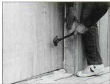
5 Wall stud was \frac{3}{4} in. away from rough opening, so plywood was added to fill void and provide a base for fastening door.
