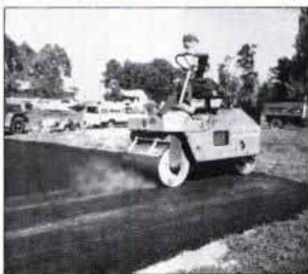
13 A 1½-ton roller compacts the still-hot, soft asphalt. Thorough compaction is one of the key steps to a long-lasting driveway.
