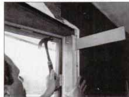
10 Fit extension jamb into pre-routed groove to build out window jamb flush with finished wall. Shim jamb, if necessary.
