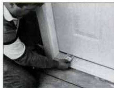
14 Test sill height with a dollar bill. Close door on bill and tug gently. If the bill can be moved freely, readjust sill for a tighter fit.
