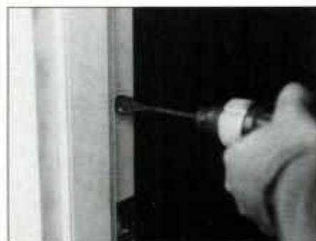
12 Mark the strike-plate location on door jamb and bore a hole for the dead bolt with a spade bit. Then, mortise the plate flush.
