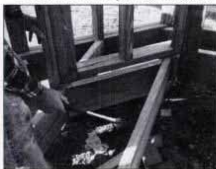
13 Add piece of 2x8 solid blocking between joists in front of angled wall. Blocking provides a nailing surface for decking.
