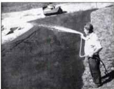
15 After it's rolled thoroughly, the driveway is sprayed with a garden hose to cool off the asphalt and start it hardening.
