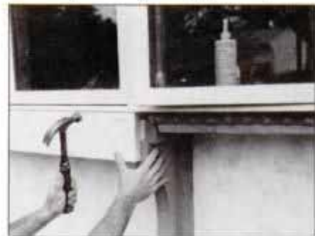
7 Nail trim boards along window bottom. Note brace bolted to wall, under center of window, to support projecting unit.
