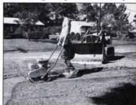
5 A gasoline-powered compactor—a flat-bottomed, ground-pounding machine—is used to compact processed stone tightly.
