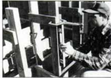
11 Screw 1x4 cross brace to outside stud. Then, plumb inside stud and clamp the brace to it. Now screw brace to inside stud.
