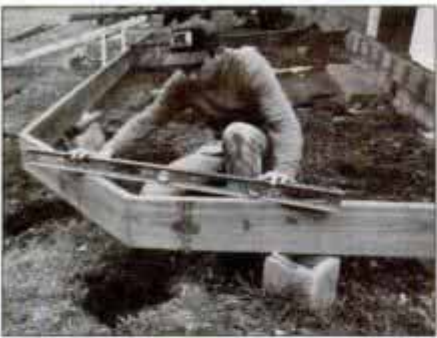
4 With header joist temporarily supported by concrete blocks, shim header level. Then, take measurements for posts.
