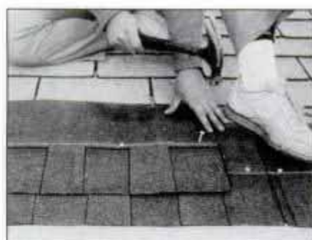
6 Align top edge of shingle with bottom edge of fourth course of old shingles. Nail in place along chalked nailing line.
