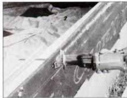
3 Remove studs and nail down a double 2x4 sill plate. Use a reciprocating saw to cut sheathing and wallboard flush with sill.
