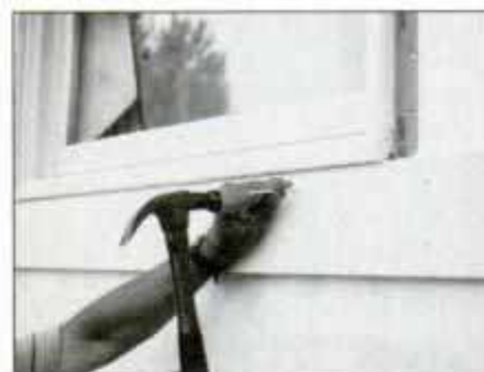
5 Nail 5 \frac{1}{2} -in.-wide pine trim under the window first. Note: Bottom trim board extends 7 \frac{1}{2} in. beyond window on each side.
