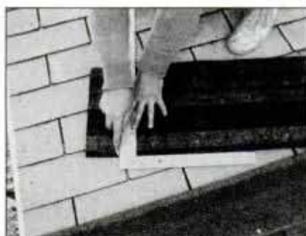
5 Turn over shingle and cut off waste with knife and framing square. Cutting back side is easier because it has no surface granules.
