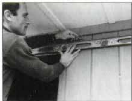
2 Use a level to mark rough opening height of new door unit. Then, draw a plumb line to establish right side of opening.
