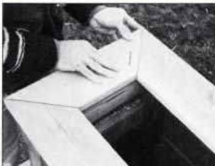
18 Finish top of the walls with 3/4 x 4 1/4-in.-wide rough-sawn cedar. Fasten cedar trim with 6d galvanized finishing nails.
