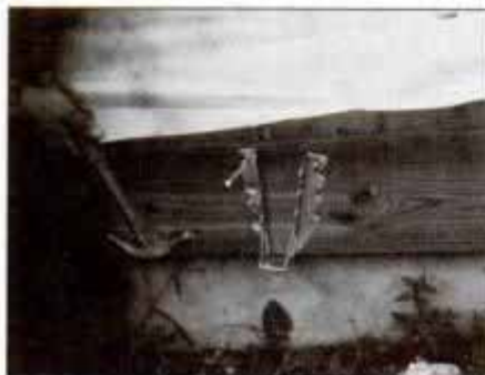
1 After bolting ledger to the house, nail metal 2x8-joist hangers 16 in. on-center. Nail only one side of metal joist hangers.
