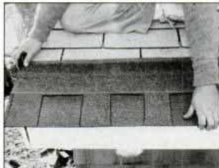
1 Begin at one roof corner with full shingle. Keep it flush with edging at rake and \frac{3}{4} in. below old shingles at eaves.
