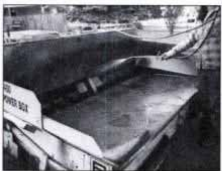
8 The paver's hopper and corkscrew auger receive a light coat of lubricating oil to prevent the hot-mix asphalt from sticking.
