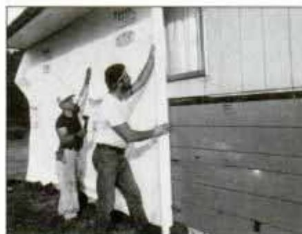
1 With the windows removed, Tyvek housewrap—an air infiltration barrier—is stapled directly to the exterior sheathing.
