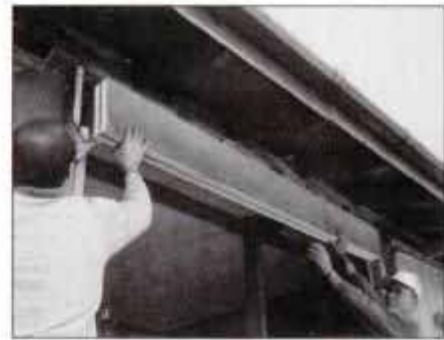
4 Install new header, if needed, for the bow window. Make header from two 2x10s separated by ½-in. plywood spacer.
