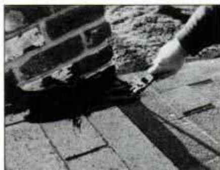
8 When you reach chimney or roof vent, cut and nail first shingle. Cover end, down to nailing line, with plastic roof cement.
