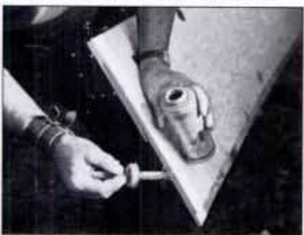
13 Use a small brush to stain all cut ends. Stain helps to seal and weatherproof the edges of shingles and plywood backing.
