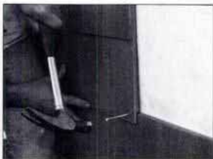
11 Position nails 1/2 in. up from bottom edge to catch both siding courses. Note rabbet cut in rear, bottom edge of siding.
