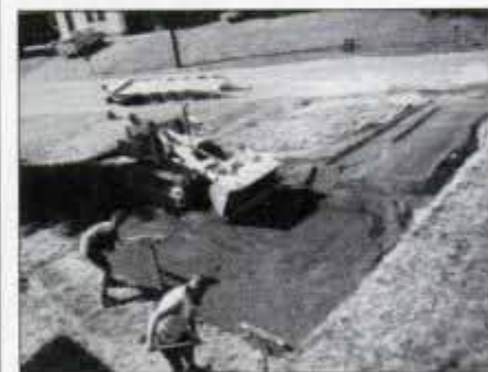
4 Man and machine work together to spread the processed stone evenly. A minimum of 4 in. of stone is required as a base.
